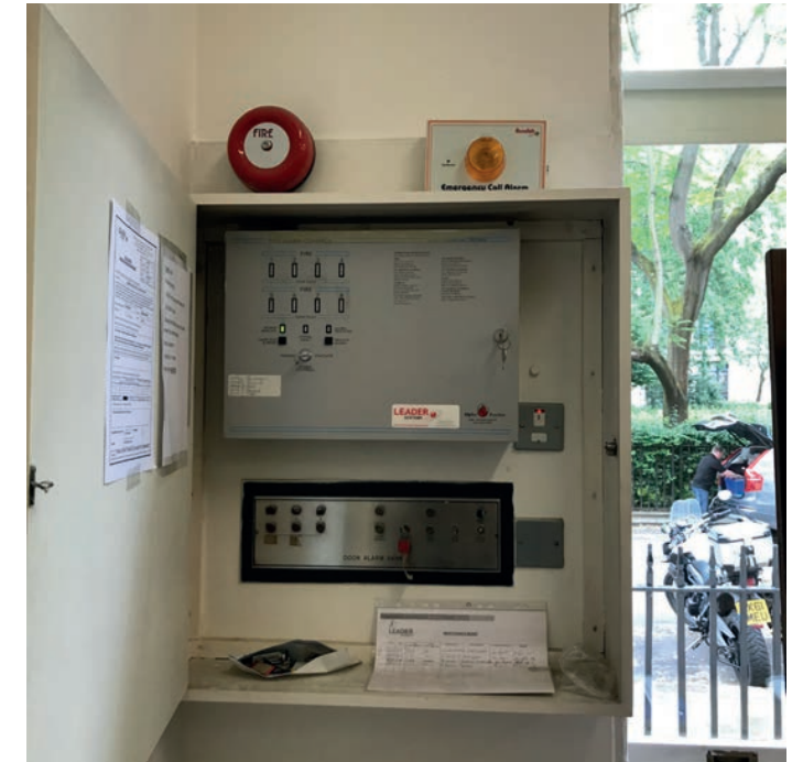
Figure 6.1 Fire Panel in ground floor reception room
