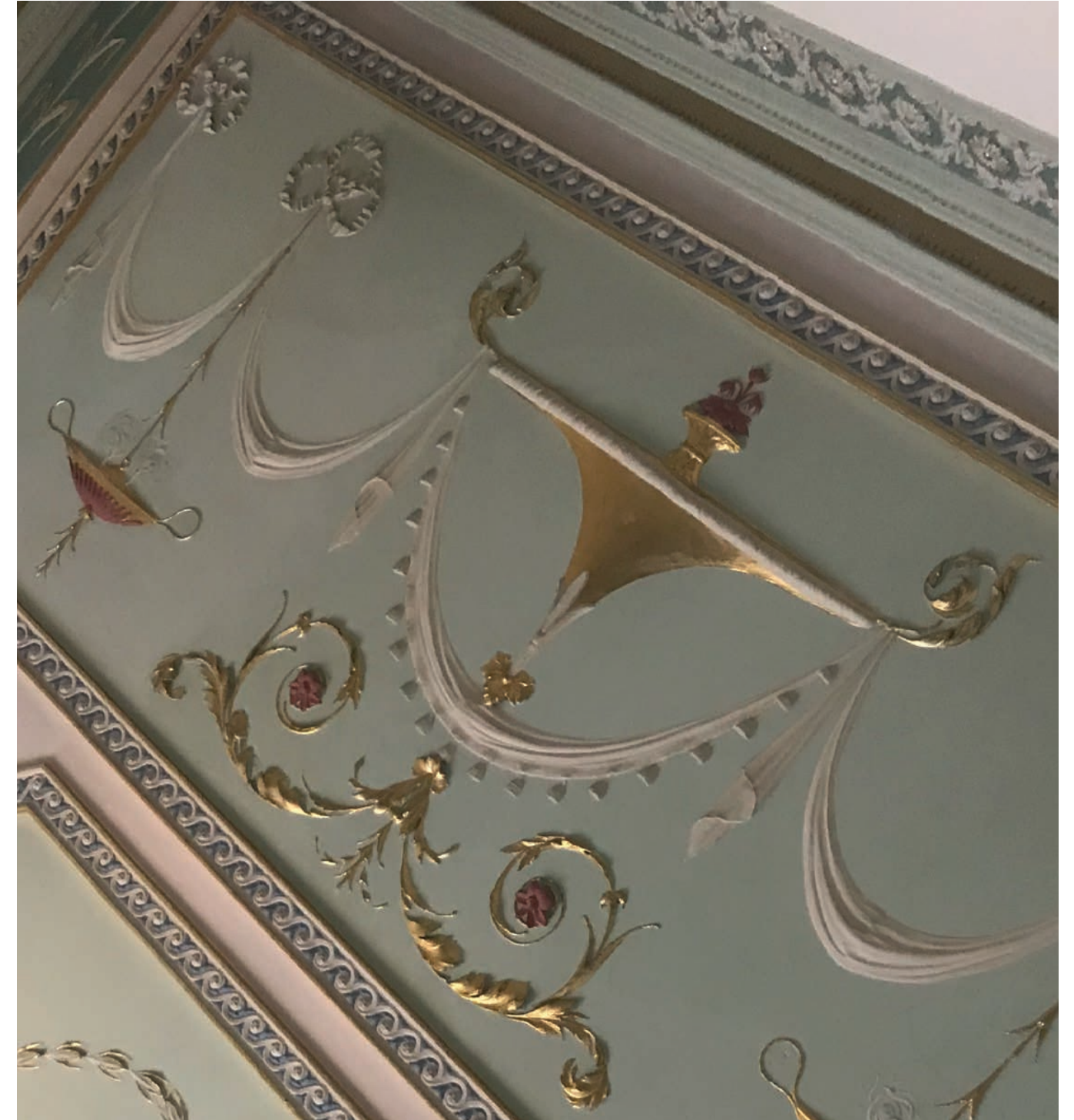
Figure 5.29 The possibly Nash / Adams Brothers ceiling in the current common room, of exceptional aesthetic value.
