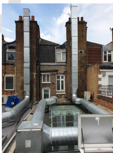
FIGURE 2: Existing ductwork and kitchen extract fan – 41 Parkway
