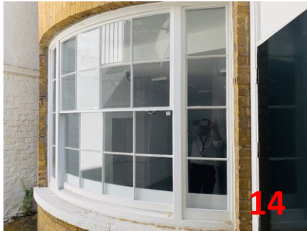
News sash window B.01.W03 Basement level of 8 MS – new sliding timber sash window to match existing rotten and damaged window
