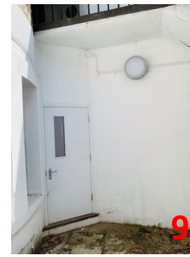
Rear lightwell 10 MS - service light installed at 2500mm h
