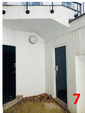
Rear lightwell 8 MS - service light installed at 2500mm h
