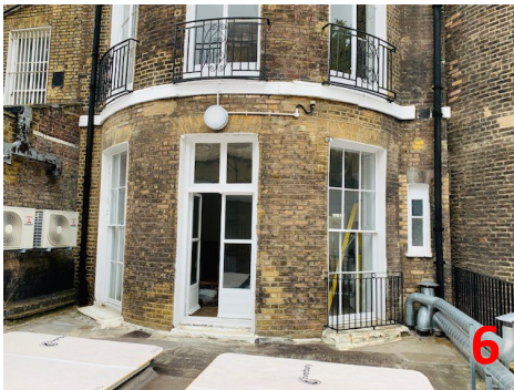
Rear of 11 Montague St - external light fitting installed to provide illumination to the ground floor terrace area, where safe access for maintenance is required to mechanical services and existing rooflights.
