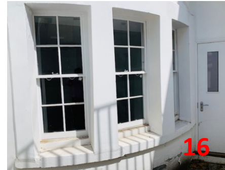
News sash window B.01.W13 Basement level of 10 MS – new sliding timber sash window to match existing rotten and damaged window
