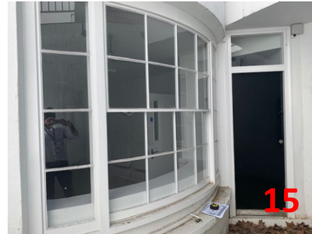
News sash window B.01.W09 Basement level of 9 MS – new sliding timber sash window to match existing rotten and damaged window
