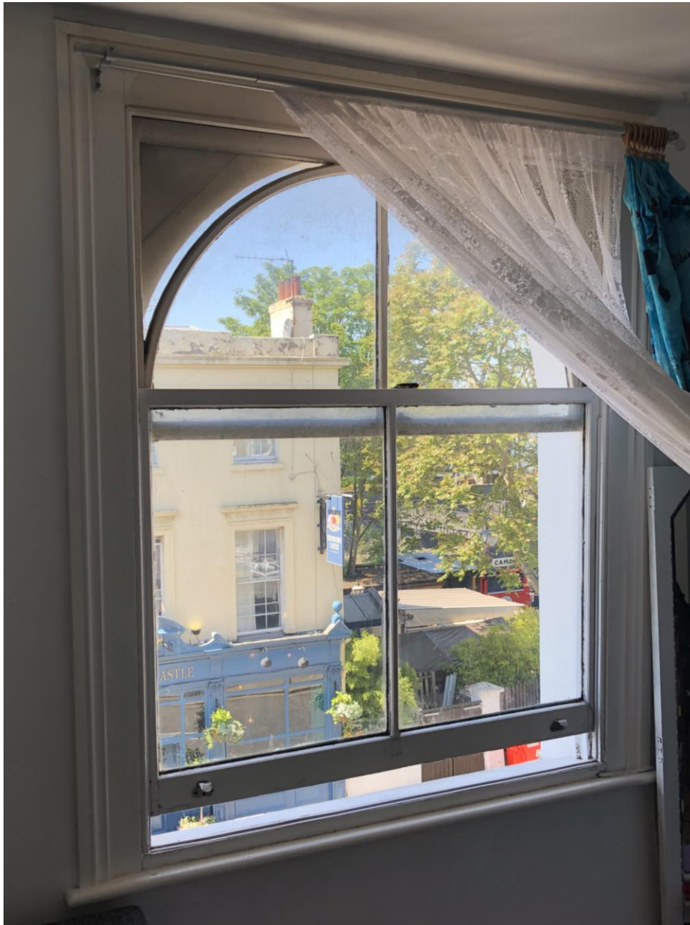
Figure 5: Internal view of window at second floor level – lounge (Flat C)
