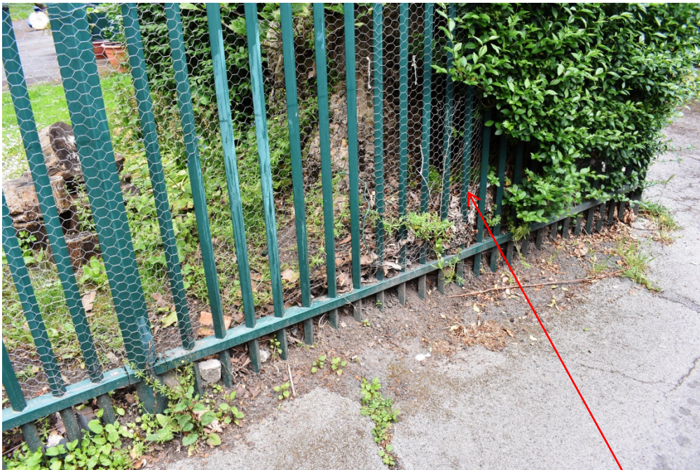
Plate 3: Detail of ground conditions of footpath adjacent, south of T1. Palisade to be removed, services installed and ground remade to suit access purposes.
