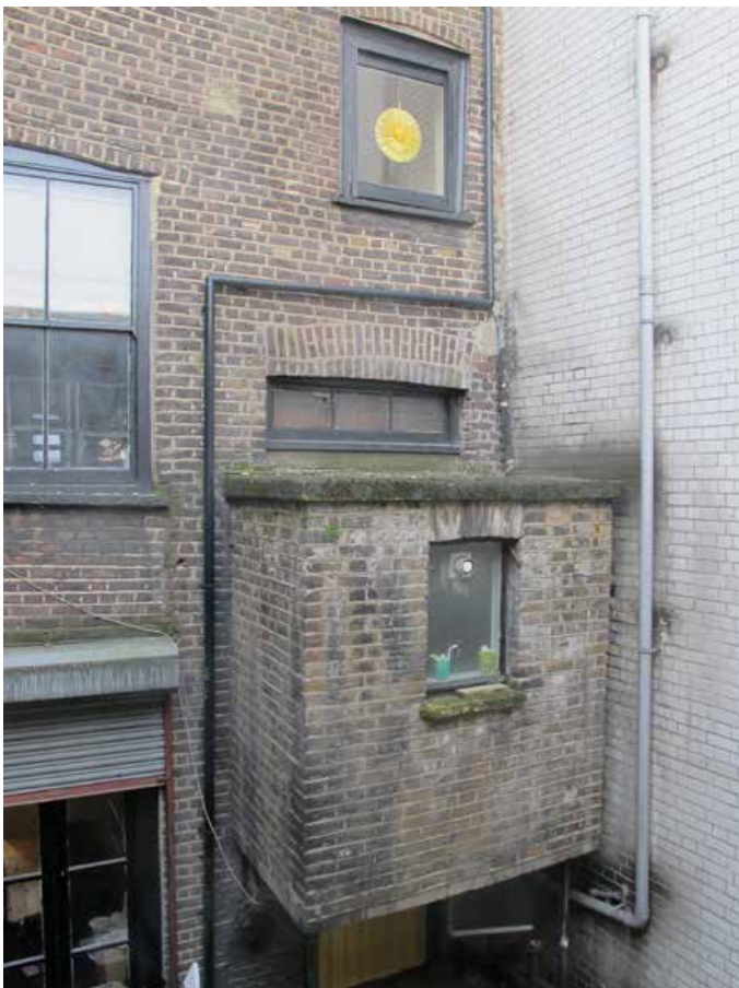
Fig. 14: View of the back elevation of No. 20 Denmark Street. The WC enclosure is a nineteenth-century addition that was rebuilt in the twentieth century
