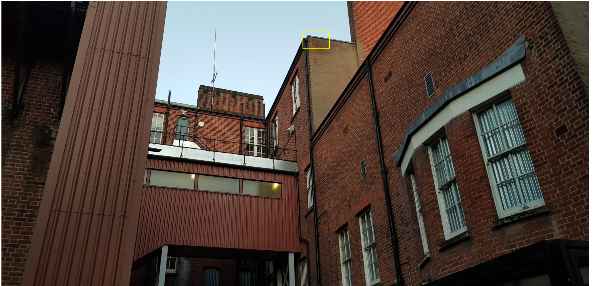
Figure 1: The north-eastern elevation of B1, showing location of common pipistrelle emergence from under lead flashing at 21:31 on 04/07/19.
