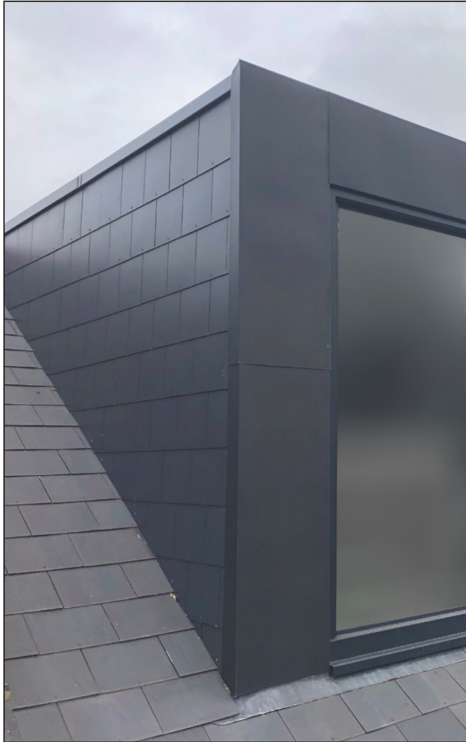
Recently completed new dormer to a house in Talbot Road, Highgate with slate tiles to dormer cheeks, to match the character and context of the existing building.
