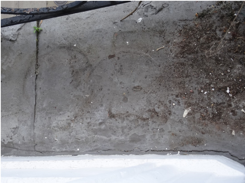
Looking down onto the balcony from the French window. There is a crack in the bituminous waterproofing of the balcony slab at the face of the wall. This may indicate that the slab has broken at the face of the wall.
