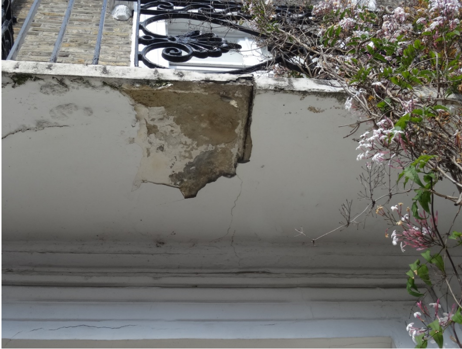
The right hand stone has dropped relative to its neighbour and a piece of stone and possibly some plaster has spalled off the bottom of the stones. Photograph taken before the prop was put in
