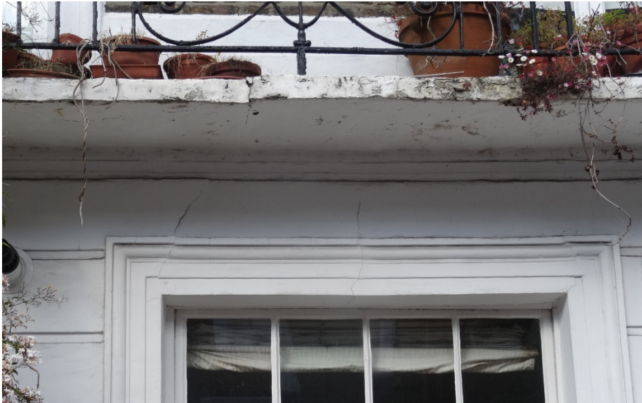
Cracks in the stucco over the Ground Floor window
