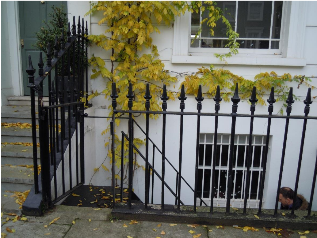
3. Front lightwell railings
