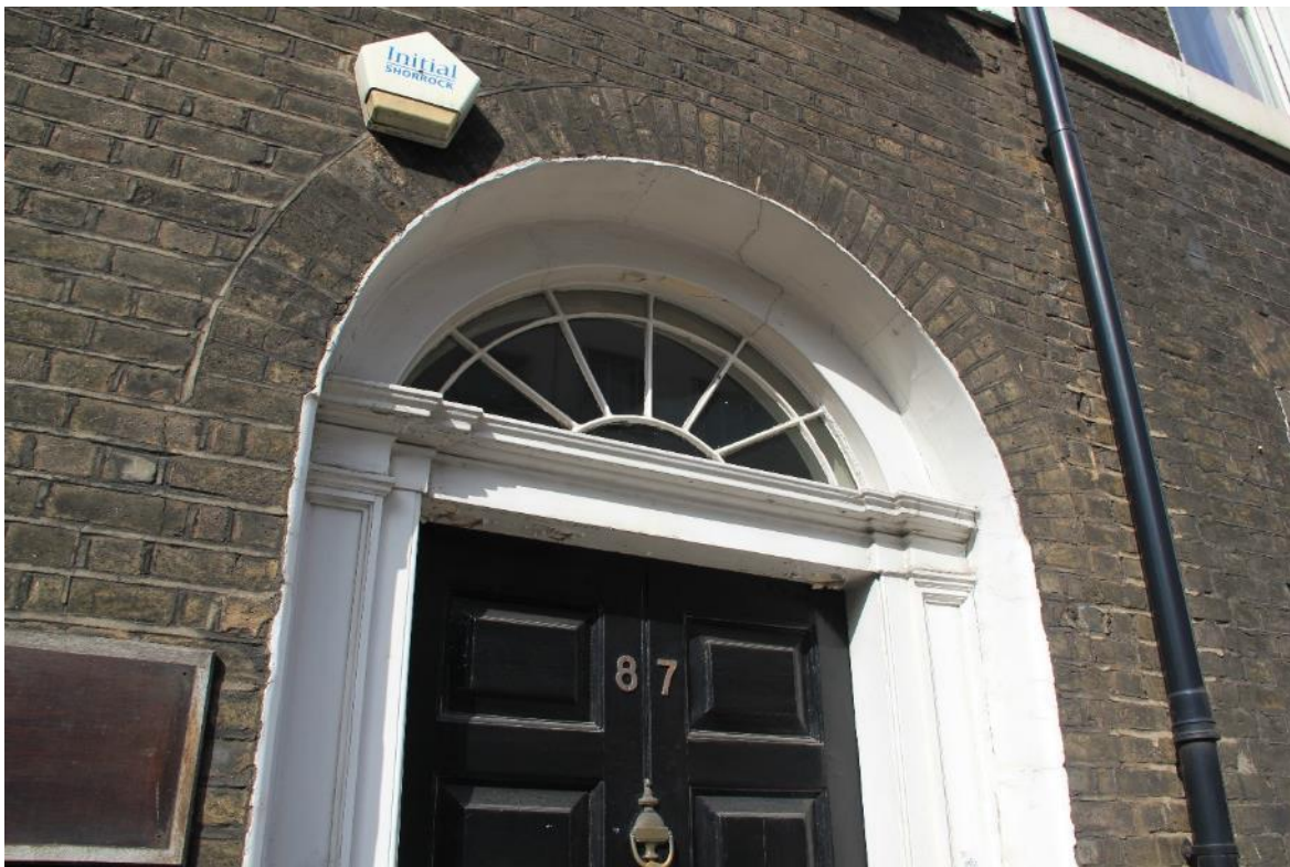
Image EDP 2: Detail of the main entrance of Number 87 showing the fanlight and moulded door frame.
