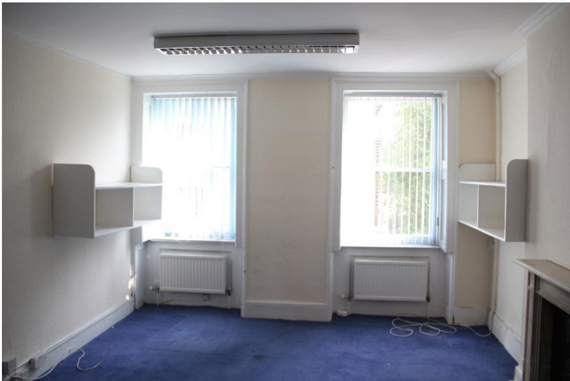
Image EDP 31: View eastwards in Room 2.2. The left-hand partition is a modern insertion.
