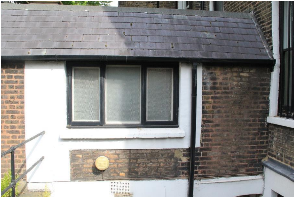
Image EDP 7: View of the single storey rear extension, showing possible extensions, looking north.
