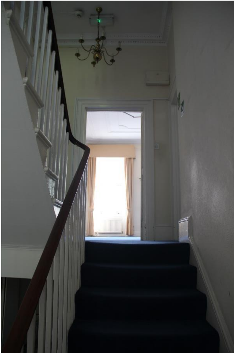
Image EDP 25: View east towards the first floor landing, showing the decorative cornice.
