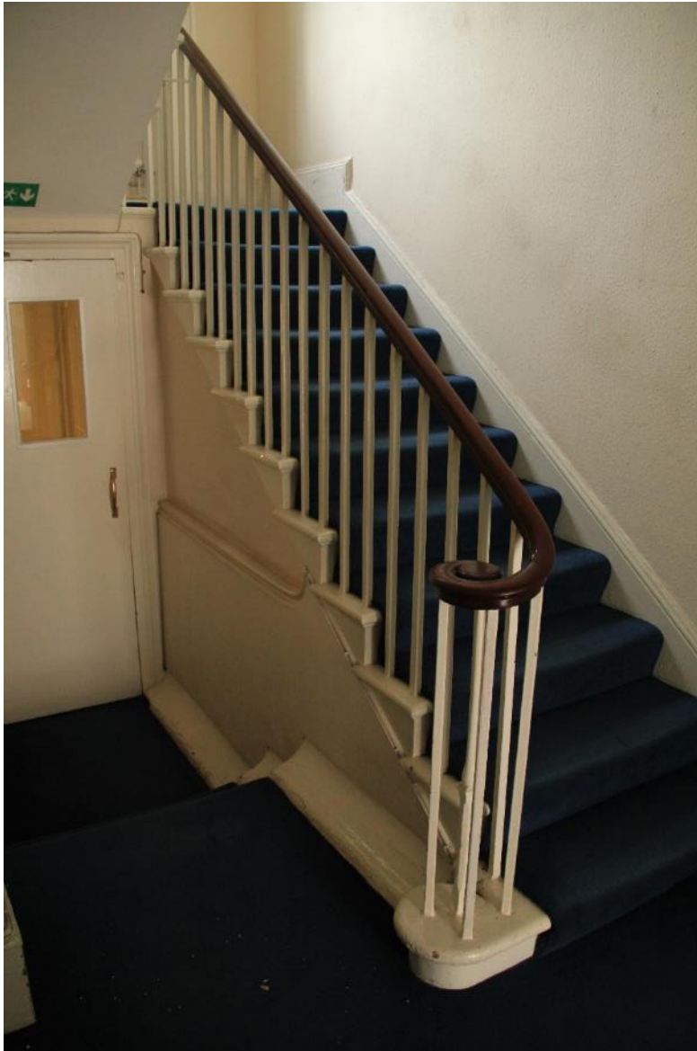
Image EDP 23: View looking north-west toward the stairs from the entrance lobby G.1 to the first floor, showing a style of typical Regency date.
