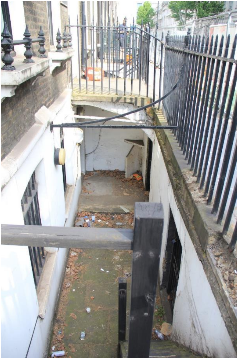
Image EDP 3: View of the front lightwell of Number 87 showing the external treatment of the basement area, looking north. The under-pavement vaults are to the right.
