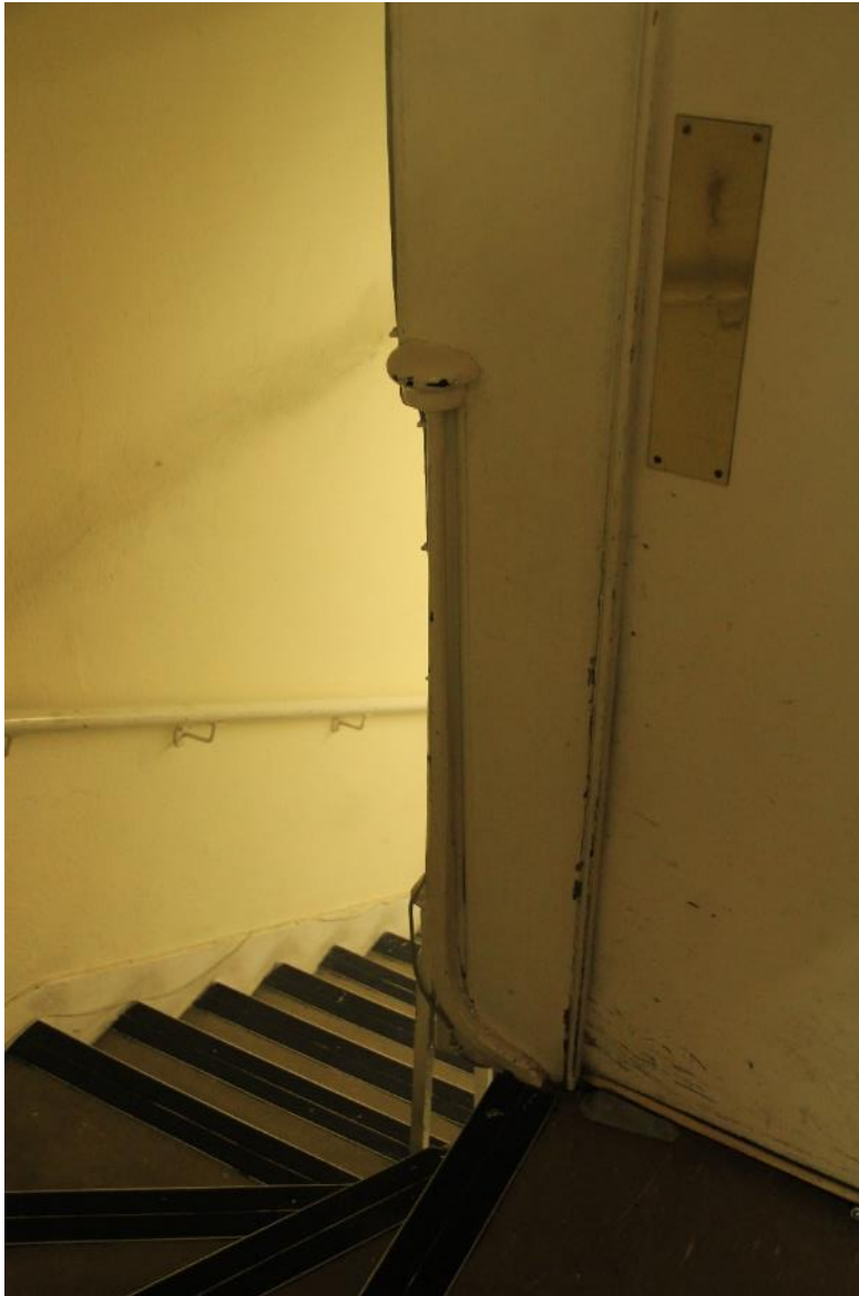
Image EDP 17: View east of the stairs down to the basement, showing the inserted fire door to the right, and the suggestion of infilled balustrade.
