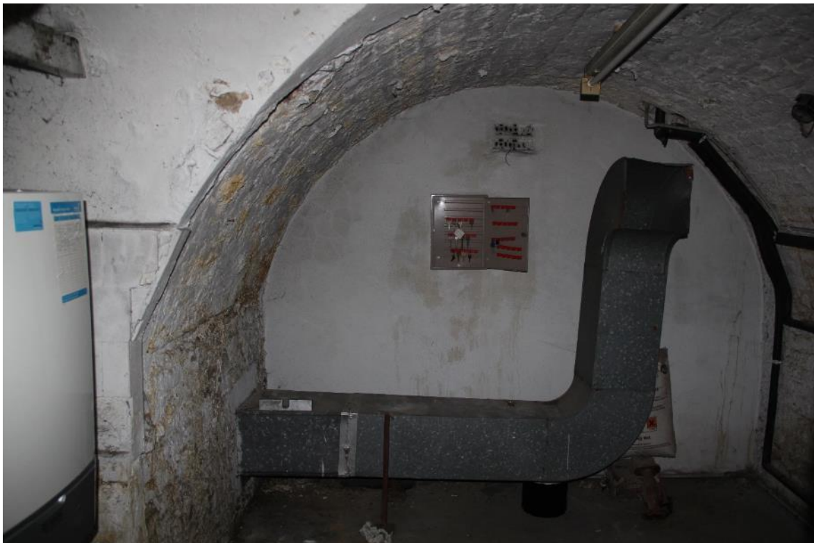
Image EDP 22: View looking west of boiler room B8 showing brick arched vault. The boiler to the left is located within a blocked doorway.
