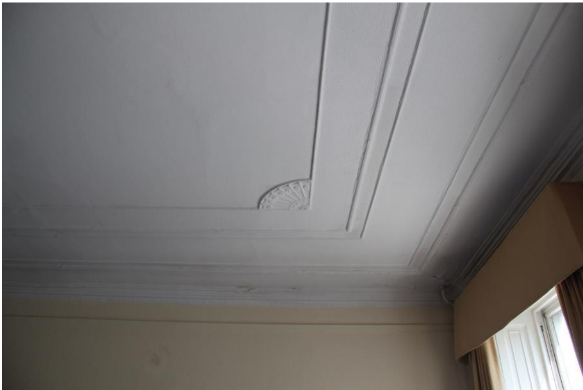
Image EDP 27: Detail of the plasterwork on the ceiling of room 1.1 looking north.
