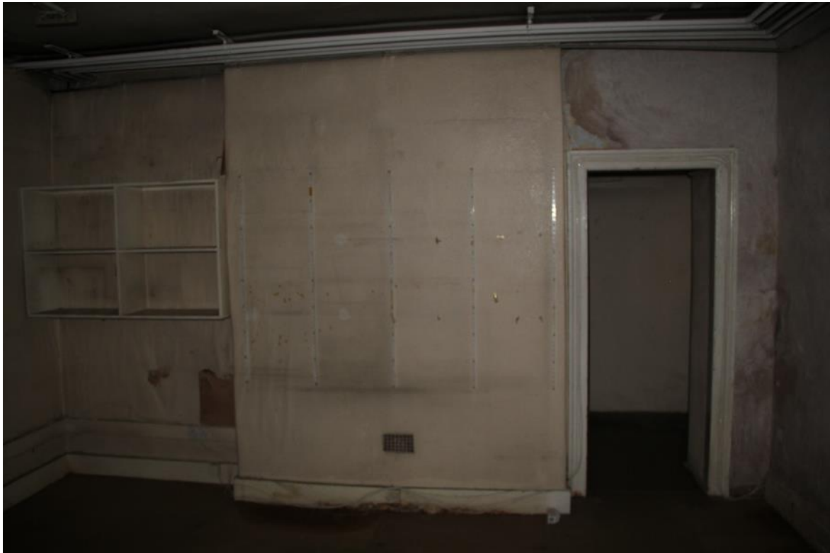
Image EDP 21: View looking south within the plain rear basement room B5, showing plain features and blocked fireplace.
