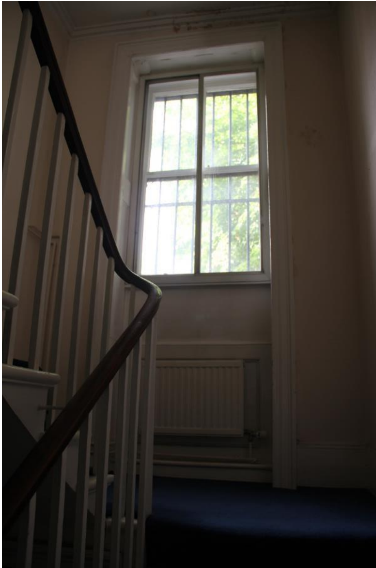
Image EDP 24: View looking west to the half-landing of the stairs, showing the plain panel beneath the window that corresponds with the roofline of the rear extension.
