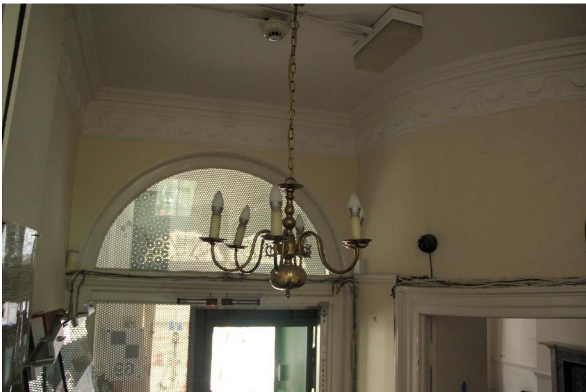
Image EDP 10: View of entrance hall G1 looking west from the stairs, here showing the nature of the cornice running around the outer wall of G.2.
