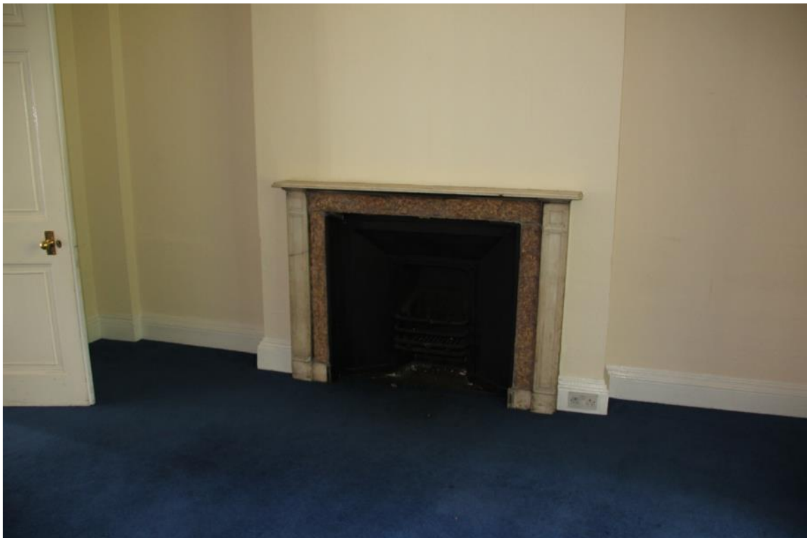
Image EDP 29: View looking south towards the fireplace in Room 1.2 at the rear of property, showing the Regency style surround and 19 th century grate.
