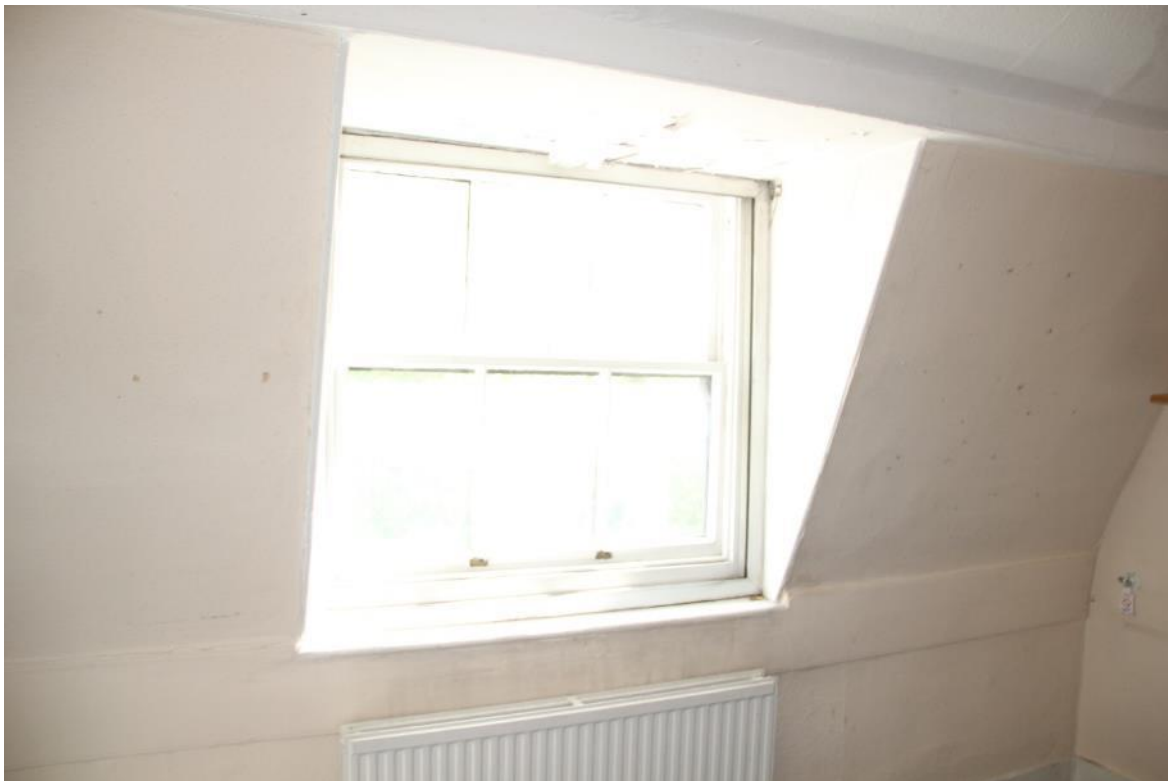
Image EDP 36: View looking east in Room 3.2, showing the broad plaster band that continues partially into neighbouring Room 3.1, indicating that the partition has been moved.
