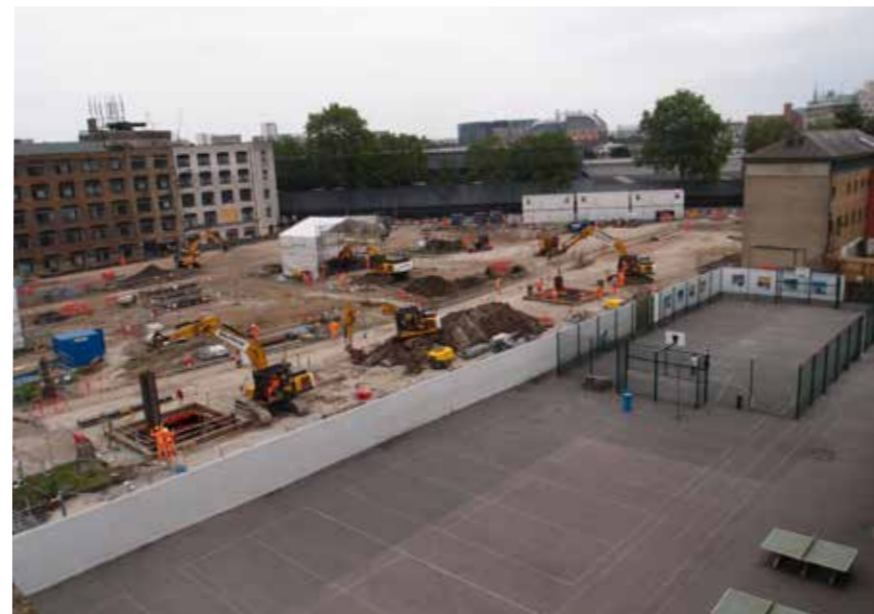
4 View from roof of existing Maria Fidelis Convent School towards the new HS2 works
