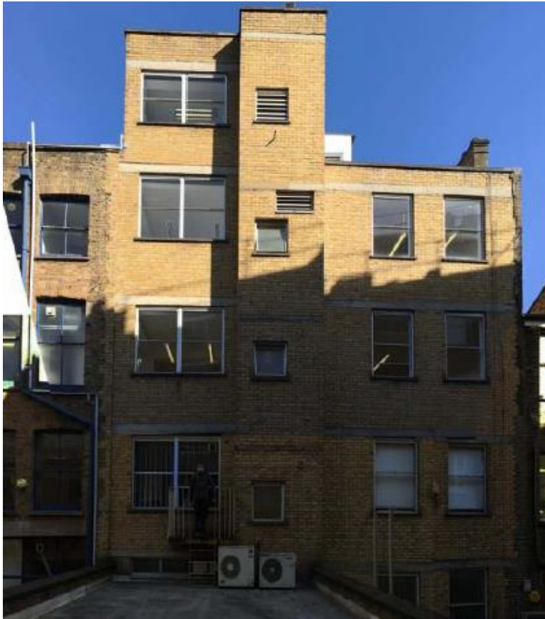
Image 3 – image of the rear elevation of the buildings (second to fifth floor level) rebuilt in the 1980s
