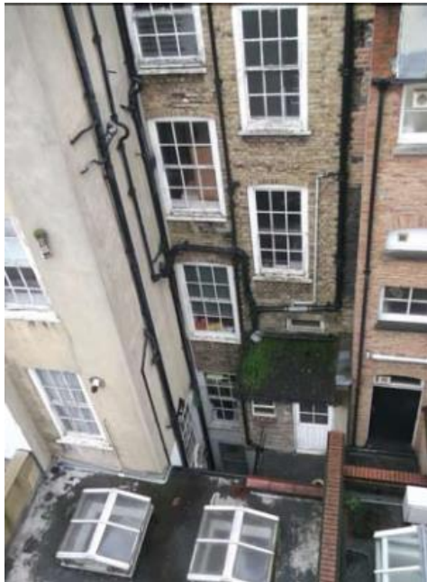
Figure 1. Photograph showing rendered closet wing and full width ground floor rear extension
