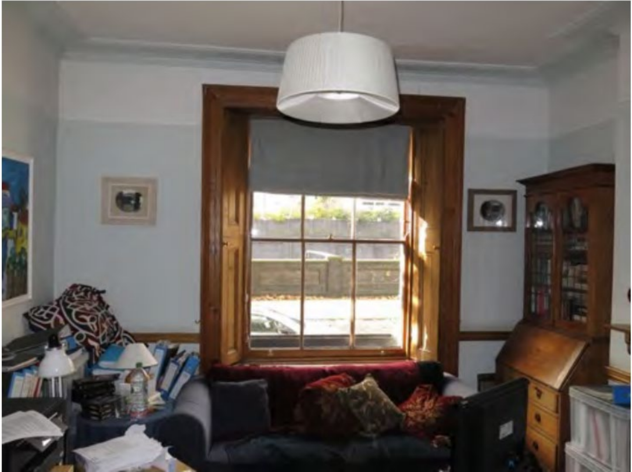
Figure 4: Internal view of external wall in the front room at ground floor
