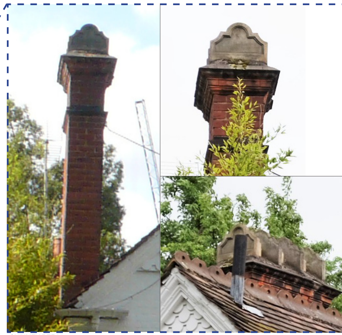
CHIMNEY REF.01 ENTIRE CHIMNEY IS TO BE RETAINED IN PLACE AND PROTECTED DURING CONSTRUCTION
