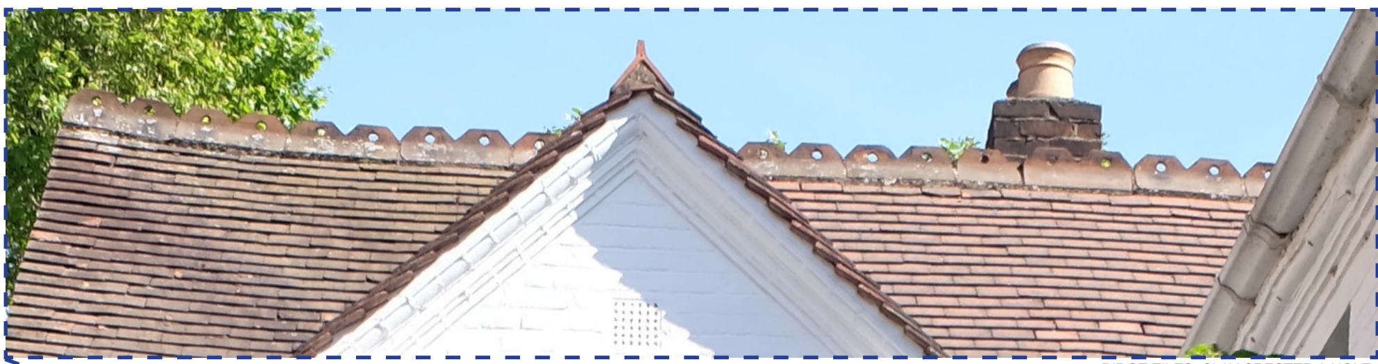
RIDGE TILES: CLAY CRESTED 2-HOLE TO BE REMOVED CAREFULLY, STORED AND REUSED. NEW TILES TO MAKE UP DIFFERENCE TO MATCH EXISTING
