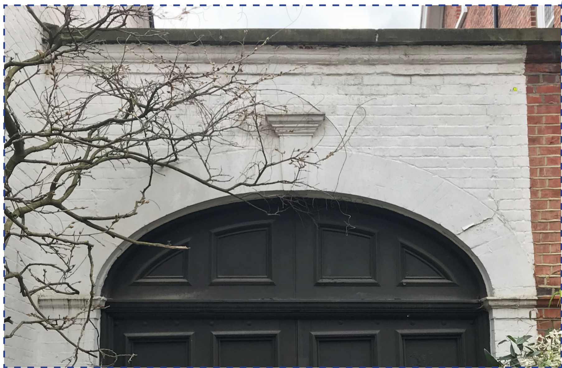
GATE ARCH & DECORATIVE KEYSTONE ENTIRE WALL, ARCH AND KEYSTONE ARE TO BE RETAINED IN PLACE AND PROTECTED DURING CONSTRUCTION
