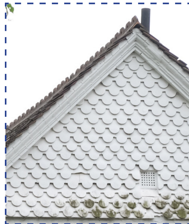
ORNAMENTAL SCALLOPED WALL TILES FACADE TO BE RETAINED IN PLACE AND PROTECTED DURING CONSTRUCTION WORKS
