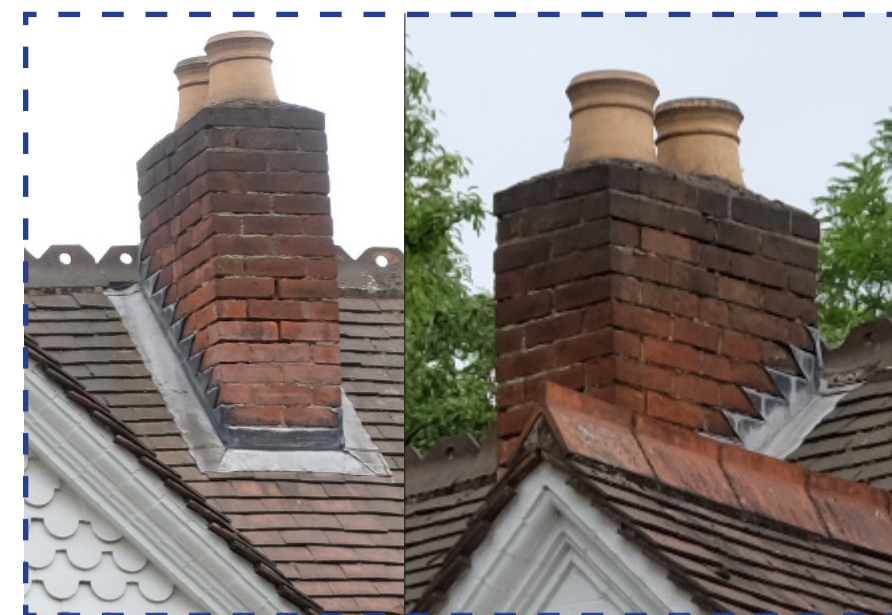
CHIMNEY REF.02 CHIMNEY TO BE REBUILT TO MATCH MATERIALS, FINISHES, CLAY POTS AND DIMENSIONS
