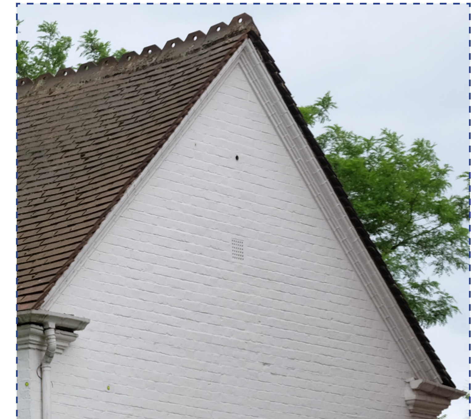
COREBELLING DETAILS AT VERGE AND EAVES DETAILING TO BE RETAINED IN PLACE AND PROTECTED DURING CONSTRUCTION WORKS
