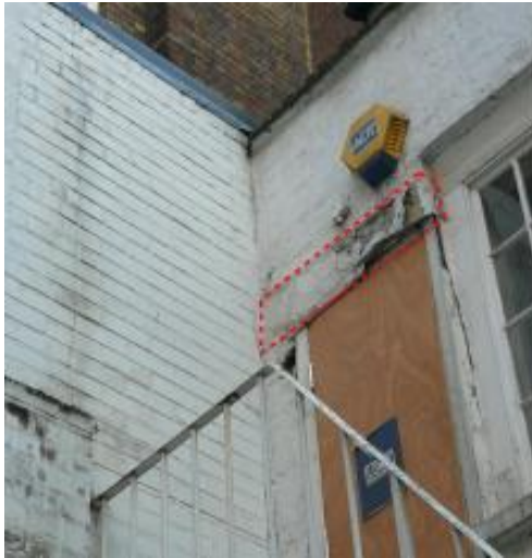
Figure 3: Decaying Timber Lintel
