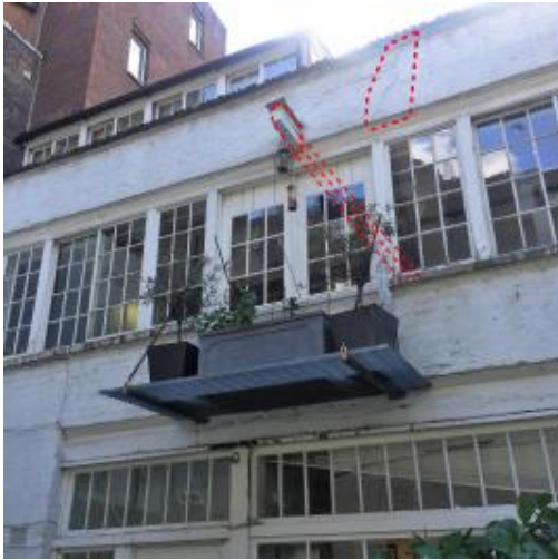
Figure 1: Protruding timber truss
