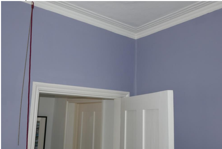
Ground floor doors, frames, and recessed book cases beside chimney breasts. Striped joinery with simple mouldings.
