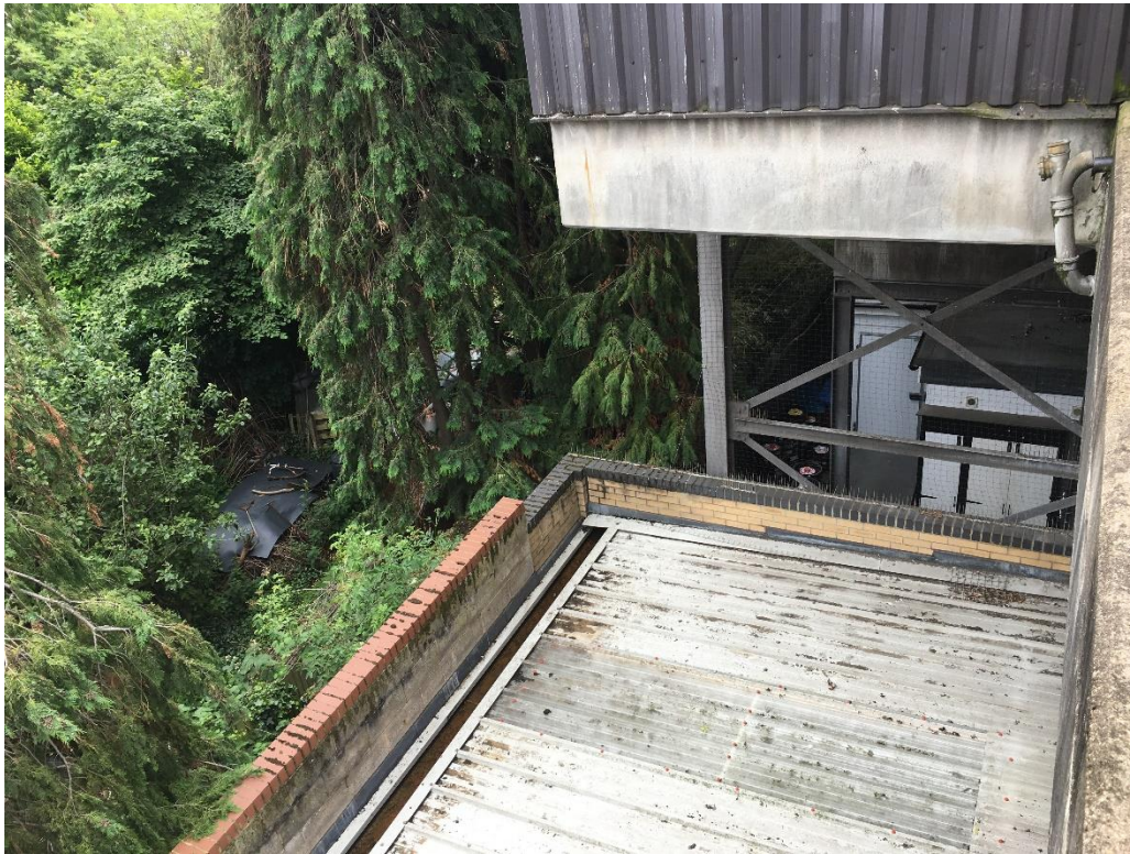
Image 6: View of storage yard to rear of Arch 55 from station platform above
