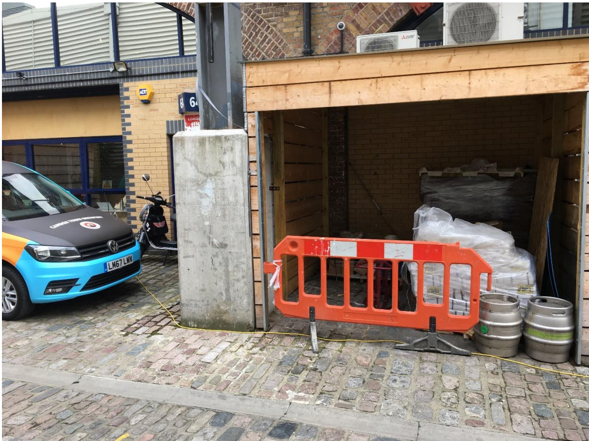
Image 7: View of tired storage sheds to be replaced with new
