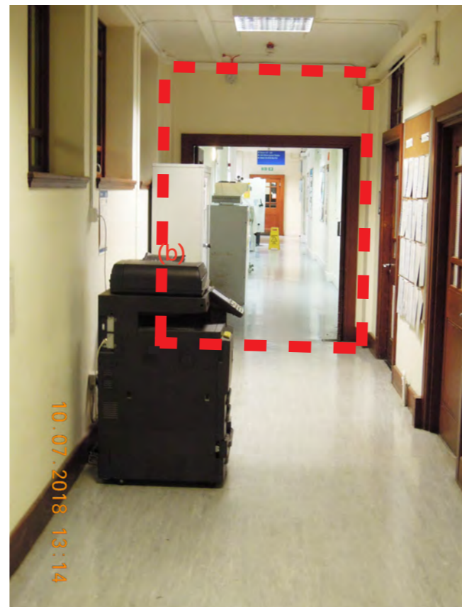
West wing N/S circulation corridor facing South showing existing door between corridor to be retained and proposed open plan future write-up space beyond
