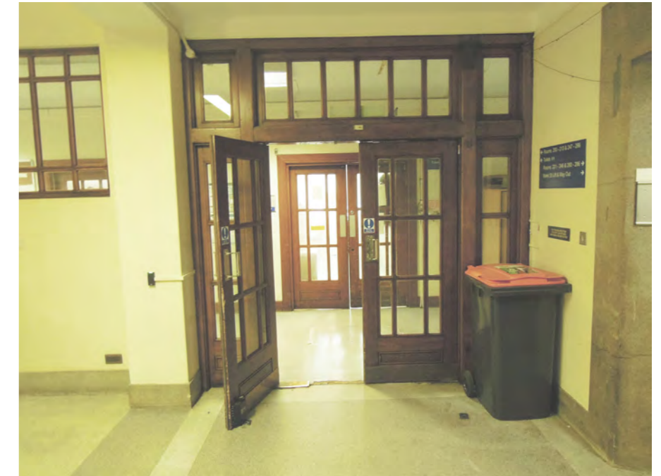
Existing Central wing west stair core and doors to be retained - view facing west
