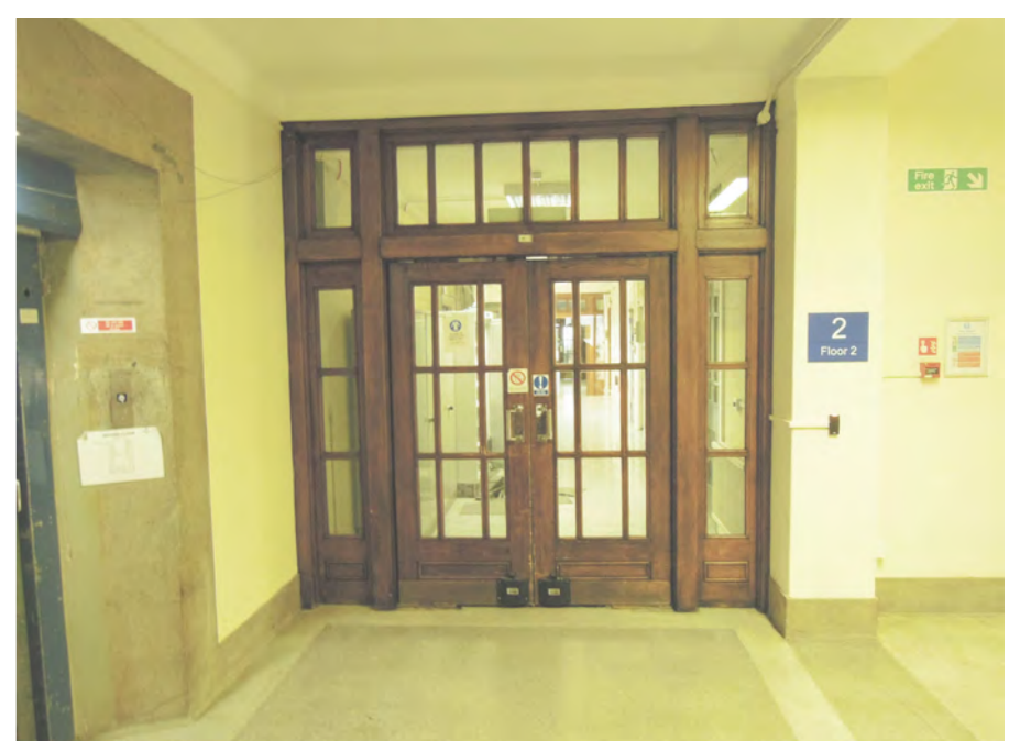
Existing Central wing west stair core and doors to be retained - view facing east Future entrance to new teaching labs
