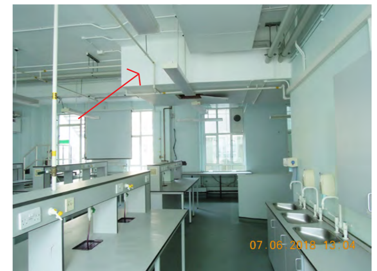
View from the teaching lab before renovation in Phase 2a, showing the exposed service trench to underside of floor slab
