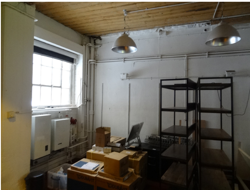
Boiles to be repositioned in G2 on a false end wall hiding pipes behind
