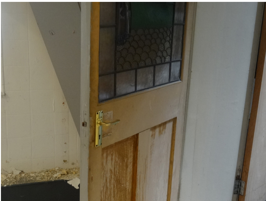
Door DG08 with modern ironmongery to be replaced
