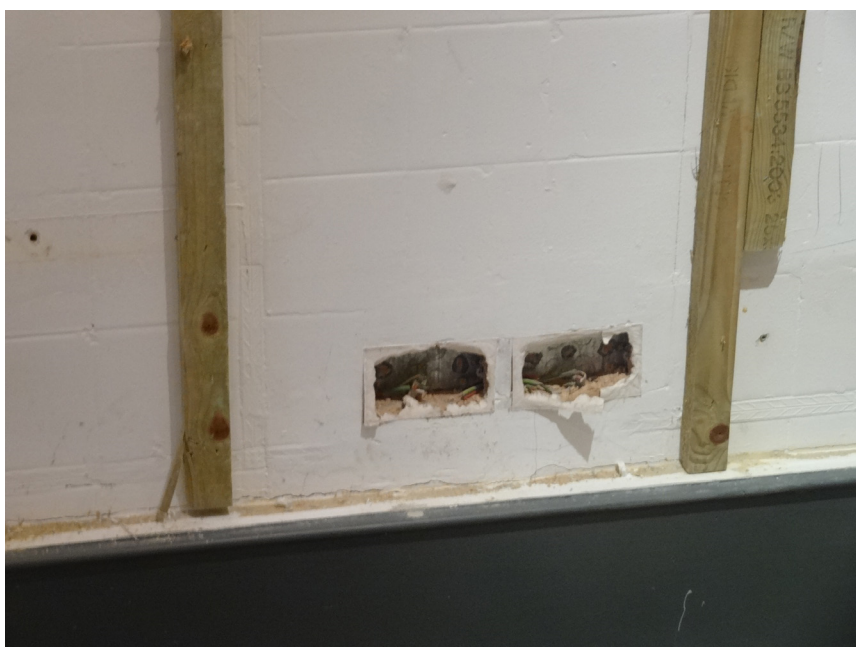
Detail from above - sockets randomly installed in original tiling
