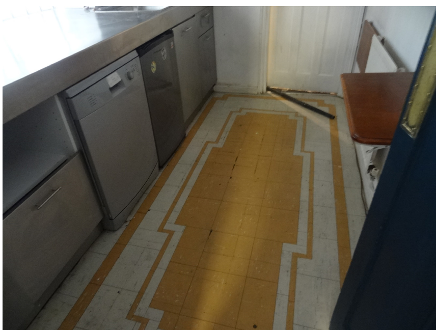
Kitchen fittings to be replaced and floor covered over
