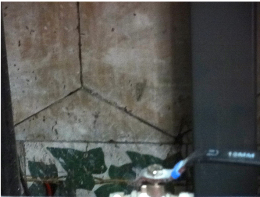
Detail of decorative tiling to be recovered after lining removed in G5
