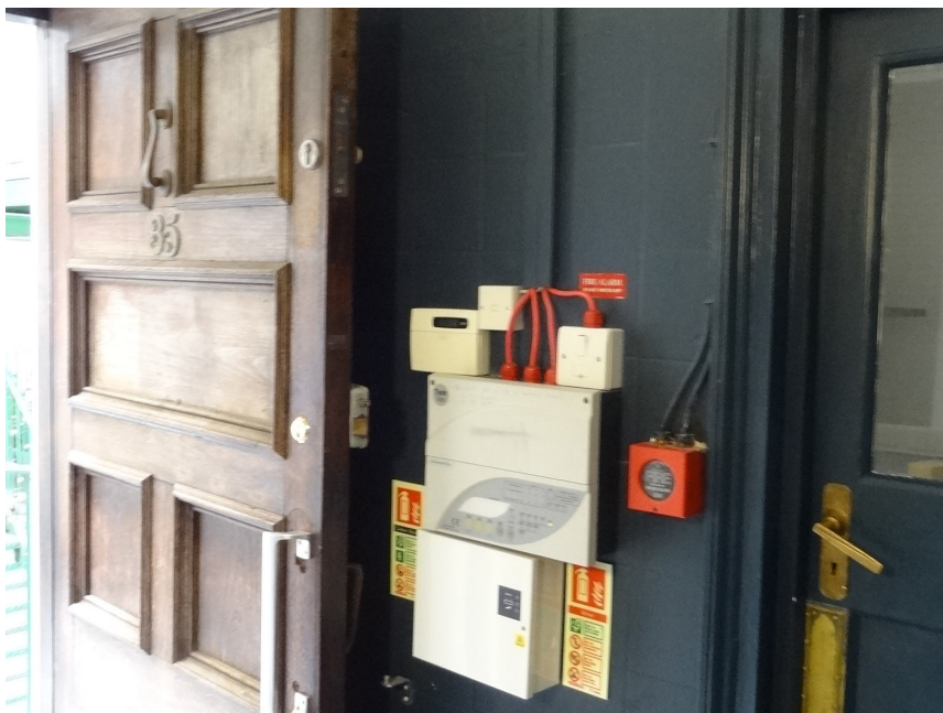
Electrics in G8 - to tidy up in a box; and exit door to open out
