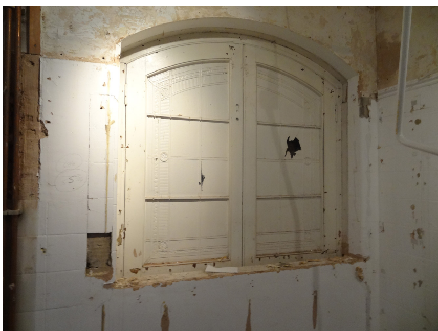
Window GW03 painted over - blocked up behind by a neighbour's wall
