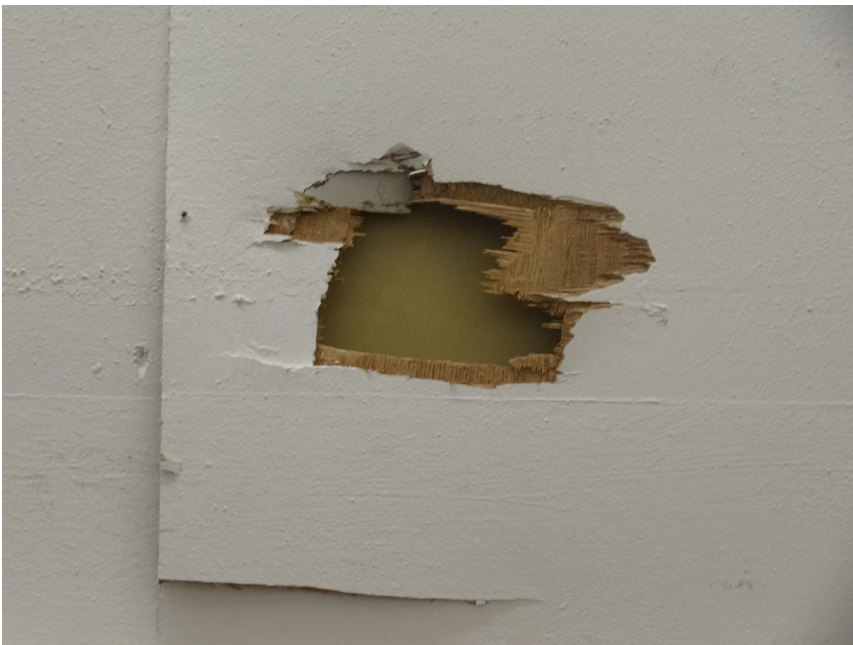
Detail of higher level lining (plastic surface behind) in G4 to be removed
