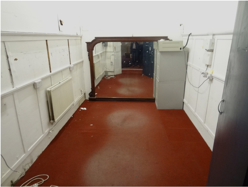
Linings in G4 to be removed, and a false floor installed above existing
