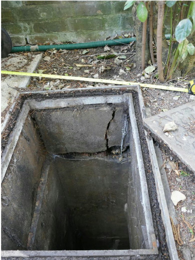
View into the drain, showing severe cracking and the base of the viburnum to the far right, as seen from this direction.
