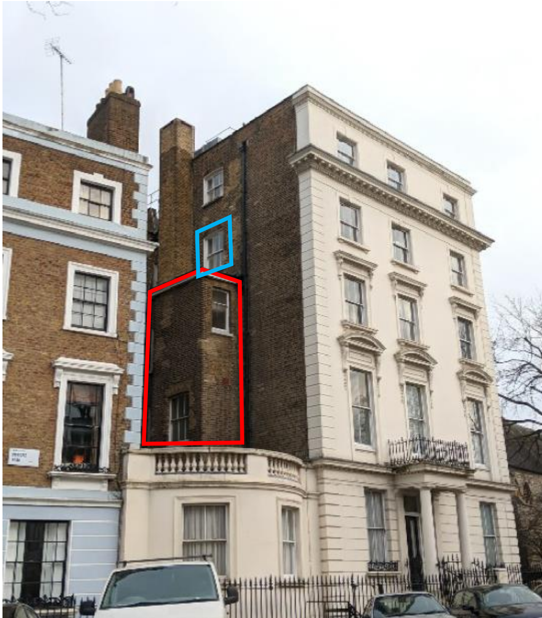
Figure 8 – The extension (indicated in red) which will have window sills lowered to accommodate new door openings. The third floor window also proposed to be altered to a door opening is indicated in blue.
