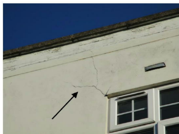
Unrelated high level render damage to left hand flank
