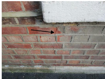
Cracking below kitchen window on left hand flank
