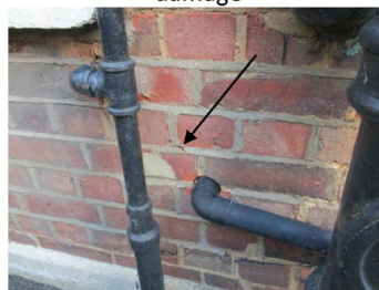
Cracking below kitchen window on left hand flank
