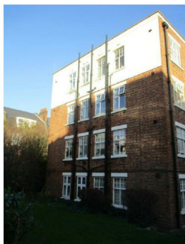
View of general area of damage
