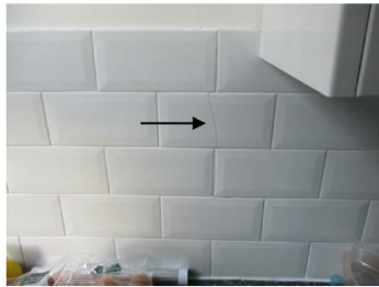
Cracking to tiles in flat 18 kitchen
