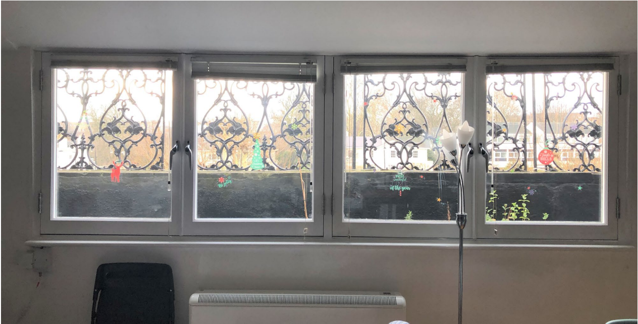
Figure 5: Internal view of the two adjacent sets of windows at third floor studio (Flat 5)
