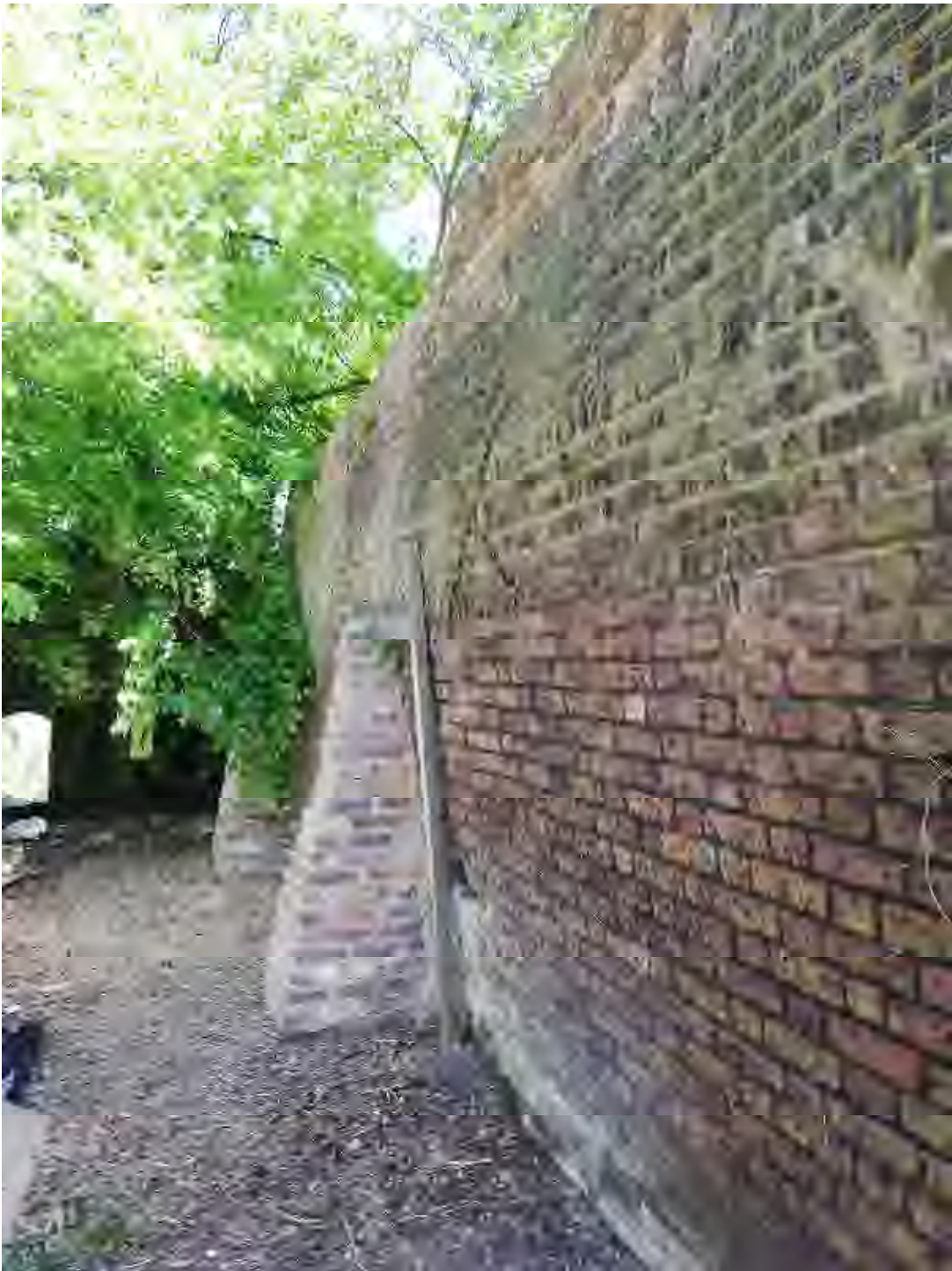
Photo 11, North Section of Wall showing newer piers and bow at the top of the elevation. Also evident is the anchor plate situated in front of the nearest pier.
