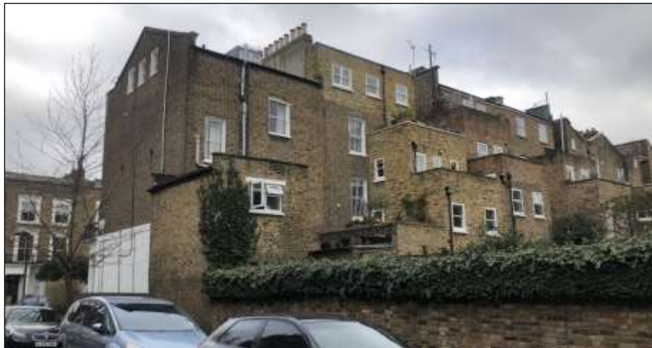
Rear of Terrace fronting Lady Margaret Road - North of the Listed Church
