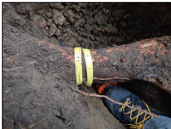
Photograph 8: Showing the largest root uncovered being 103mm in diameter.
