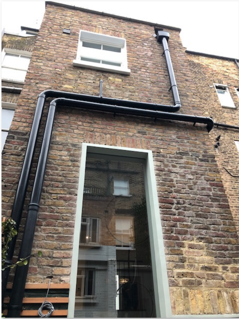
Photo 3 showing existing rear closet wing. The double height window is as existing.
