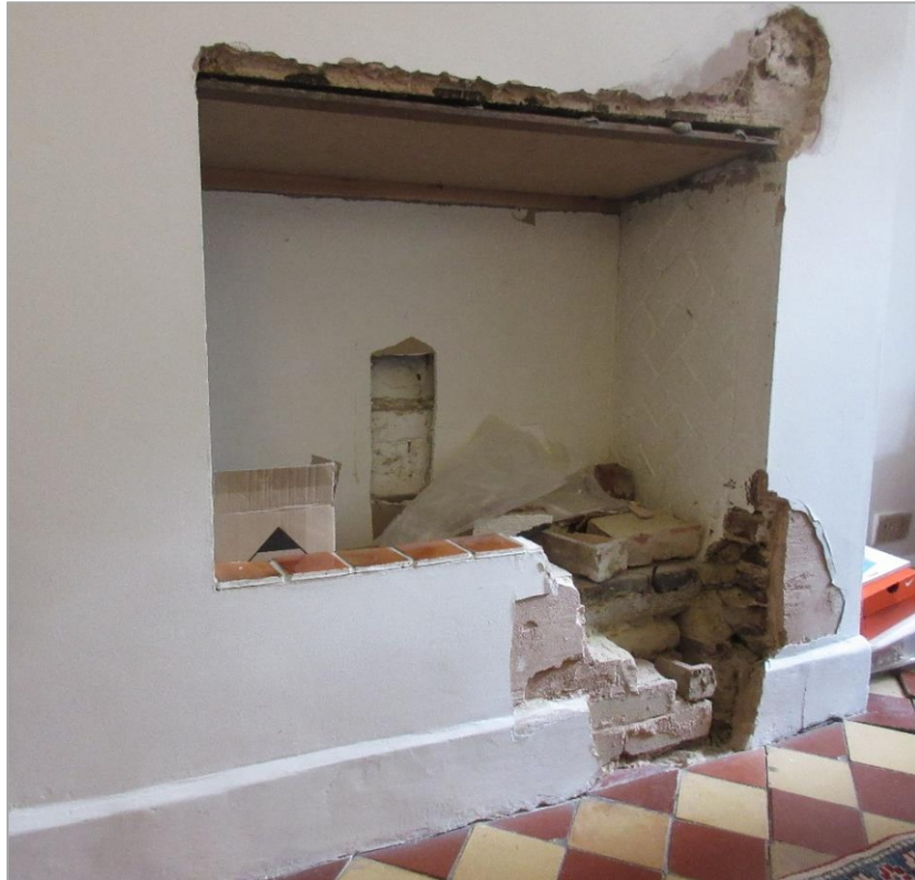
Figure 6: The dining room chimney breast has a plain opening, possibly originally for a kitchen range, with modern brick and tile infilling at the bottom
