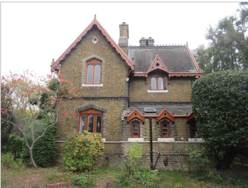
Figure 2: Side elevation, showing the lean-to roof of kitchen to right, with three gabled window heads and raised rooflight between two of these
