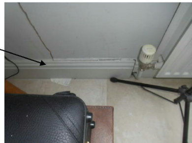
Study – separation to skirting board and crack
