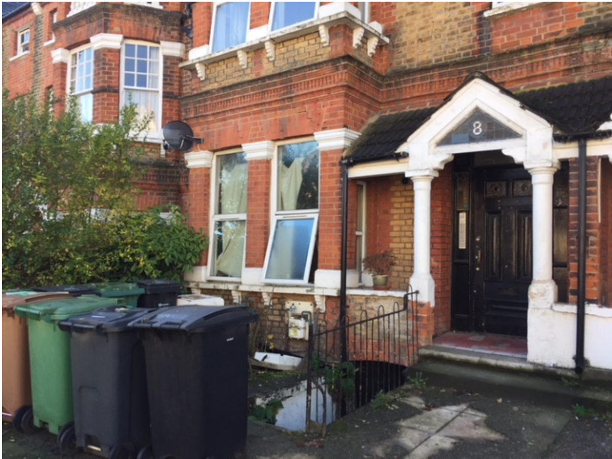
Existing front elevation and existing basement access within the front forecourt of the building
