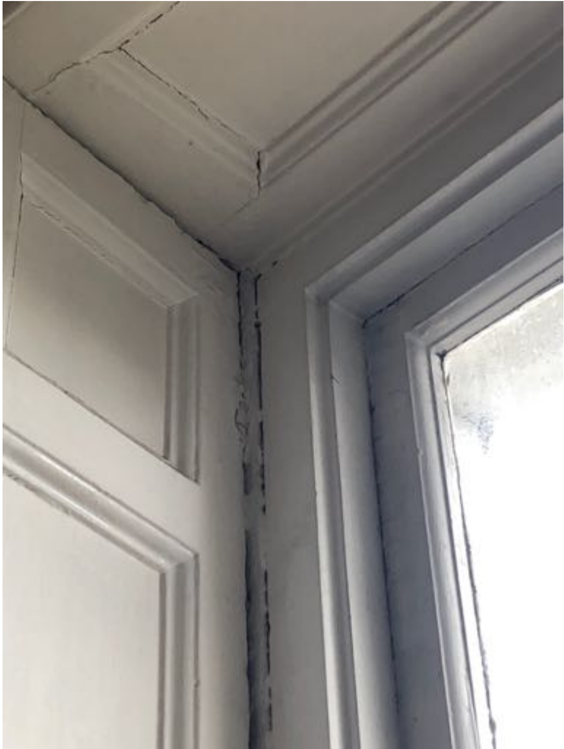
Fig 3: Evidence of existing sash – staff bead to jamb and head (second floor) Internally
