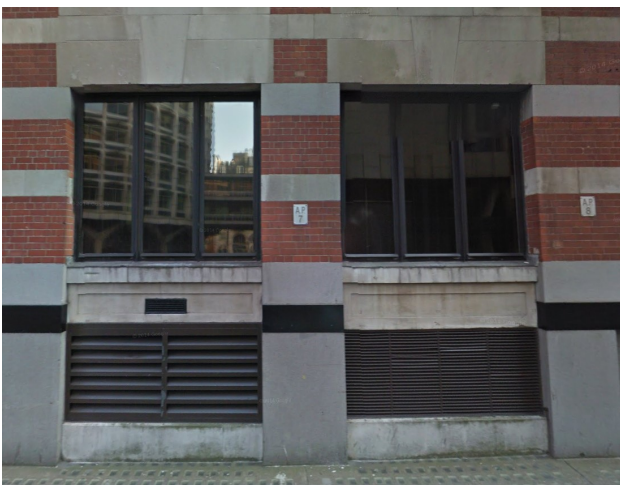
Figure 4: 2014 view of the application site, showing modern glazing to both openings and later metal louvres to the right-hand bay.
