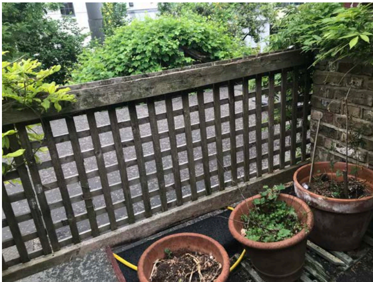
Photo 3 - View from the Terrace looking at no.4 Cliff Road shed's flat roof.
