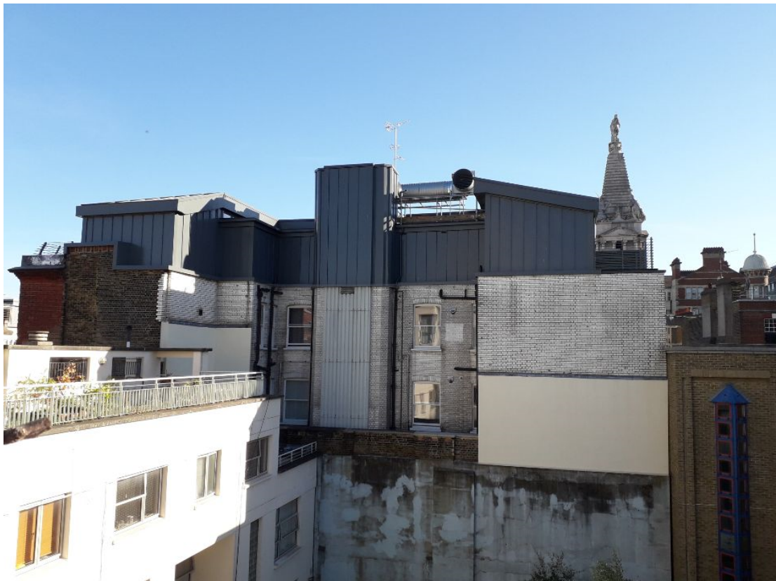
Photo 4: Unauthorised plant equipment and approved mansard from terrace across internal courtyard
