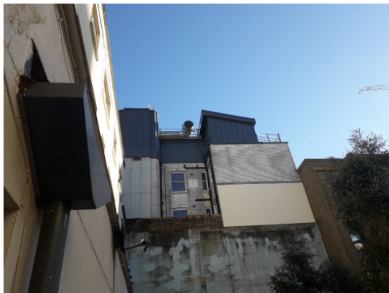
Photo 2: Unauthorised plant equipment and approved roof extension from terrace below
