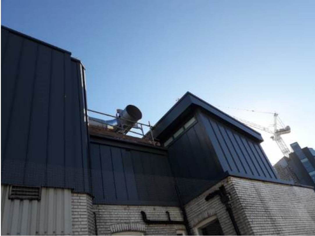
Photo 3: Unauthorised plant and approved roof extension from nearest terrace
