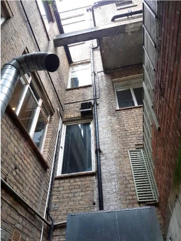
Figure 4. Rear elevation. This elevation bears little relation to the design of the front elevation. It has been extended to both sides of the building, retaining a central lightwell area. The unauthorised duct is visible on the left and is to be removed.
