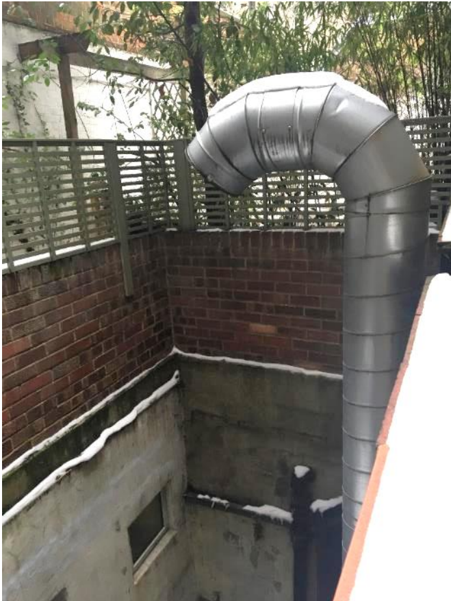
Figure 7. View of the unauthorised duct to be removed and replaced subject to receiving consent.
