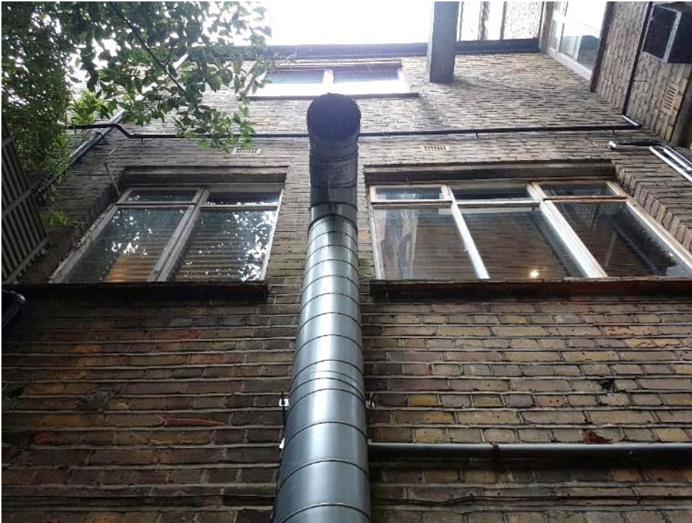
Figure 8. View of the duct be removed and replaced subject to receiving consent.
