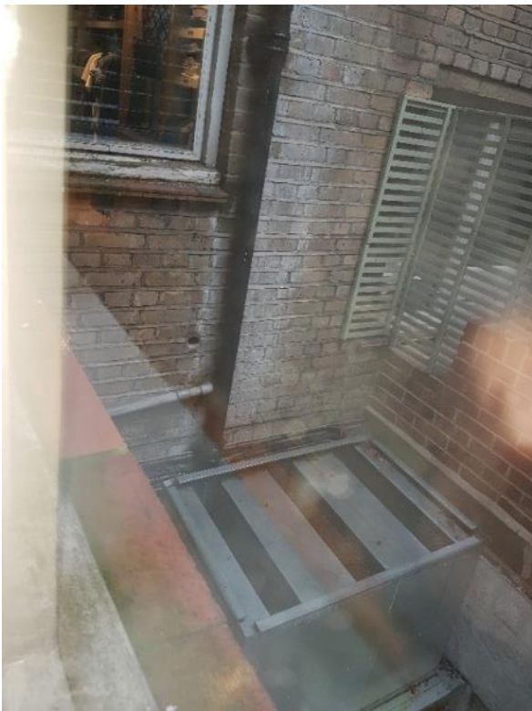
Figure 9. View of the lightwell area from the ground floor rear wing window.
