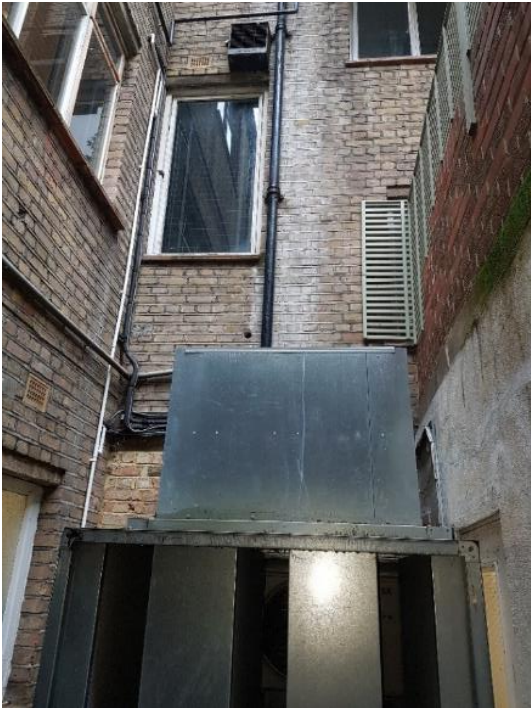
Figure 5. The unauthorised plant including attenuation housing, which is to be removed.
