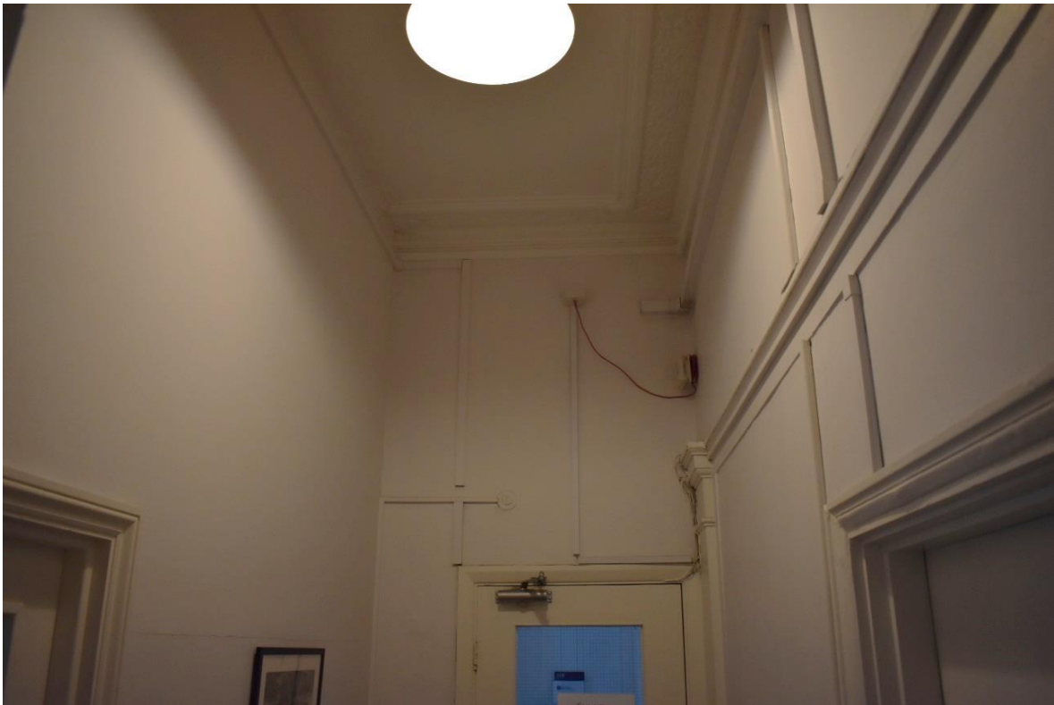
Fig 16 Two later partition walls, the right-hand one replacing an original partition, on the first floor on No.37
