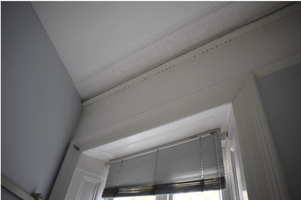
Fig 17 First floor front room of No.38, showing later partition wall cutting through original cornice
