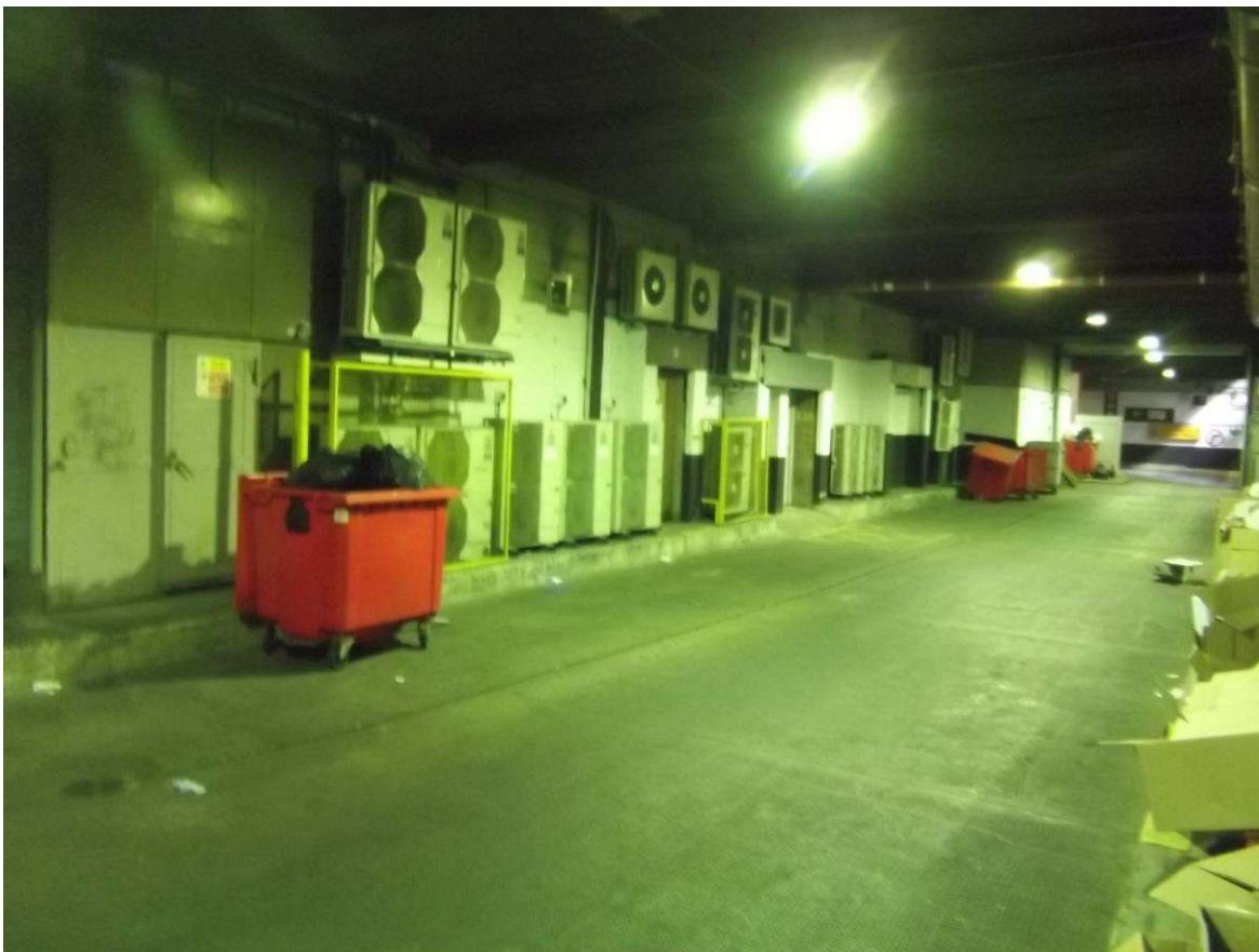
Figure 9: View looking south along service road. Note: numerous items of mechanical plant
