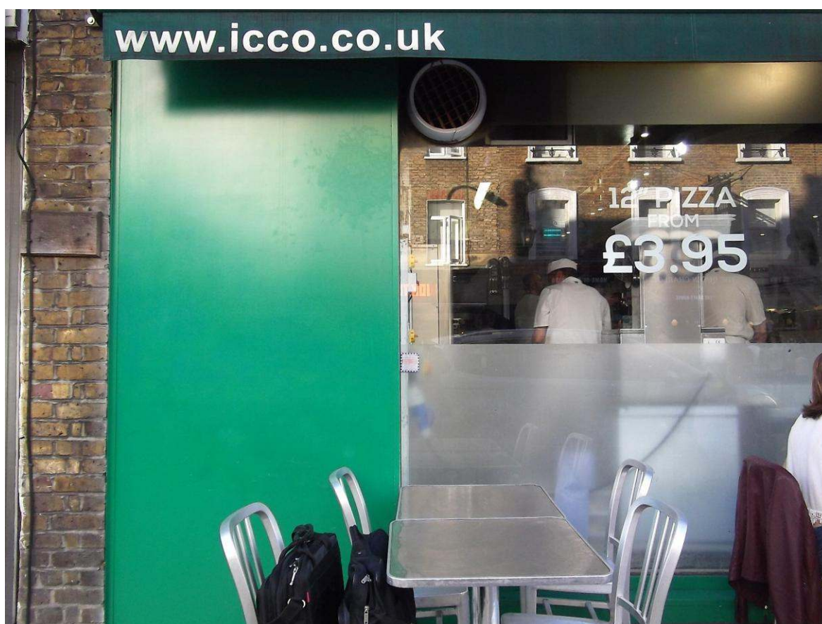
Figure 11: Oven extraction fan unit in Goodge Street façade
