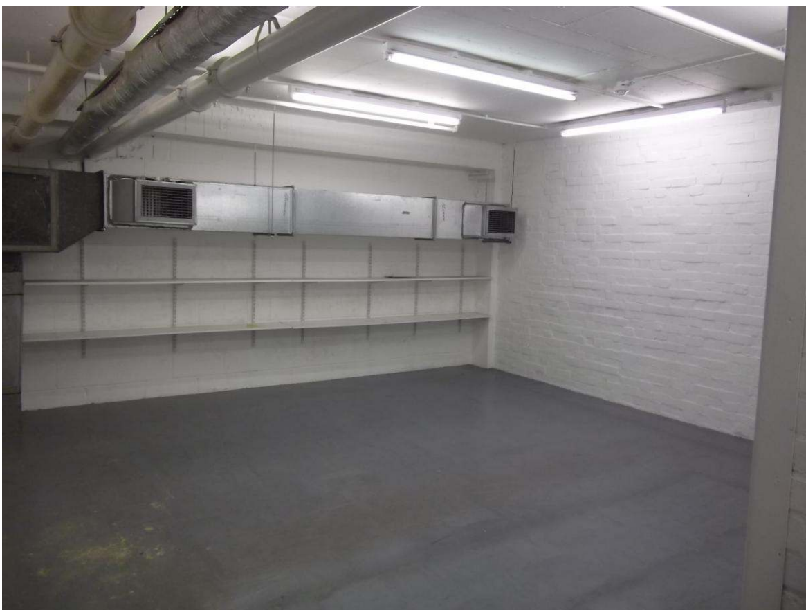
Figure 7: Mechanical air handling ductwork (existing)
