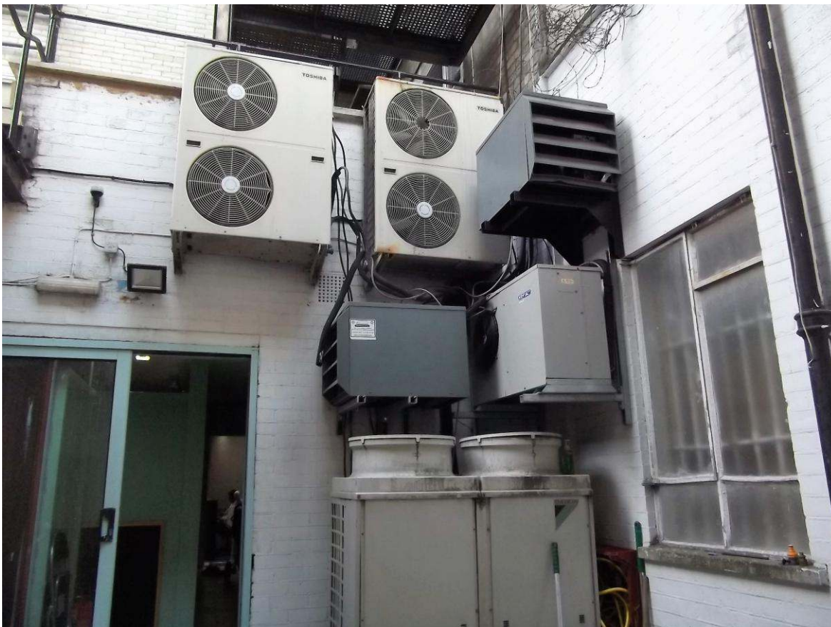
Figure 12: Air conditioning outdoor units. Note: not all items belong to ICCO. Prayer room at left of image.
