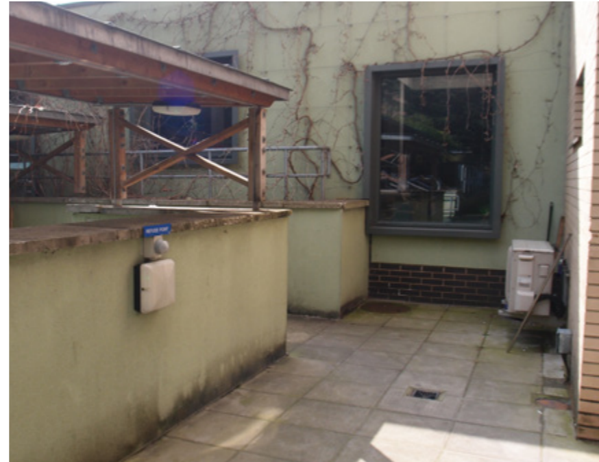
5. North elevation of commercial unit meeting east elevation of main building. Covered bin store shown to left.
