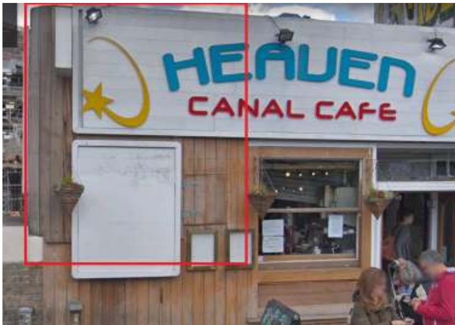
Fig 2. Existing Timber Structure over Canal Bridge Wall by which the roof is currently being accessed– Front view
