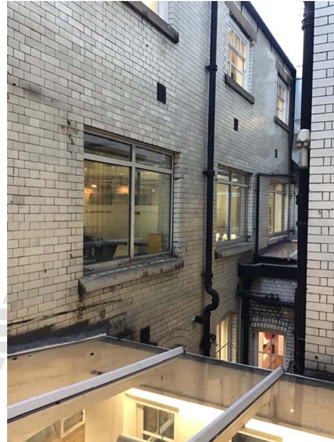
This image is in the main lightwell. The elevation shows three of the four windows proposed to be replaced. Externally walls and reveals are white glazed brick, fairfaced concrete cills and existing windows with white coated metal frames with clear double glazing as fixed lights. The lightwell continues to the basement level in the middle.
