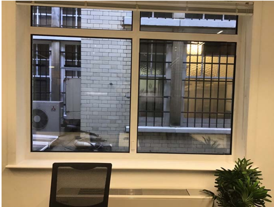
One of the windows proposed to be replaced. Internally showing boxed painted reveals, painted timber window cill.
