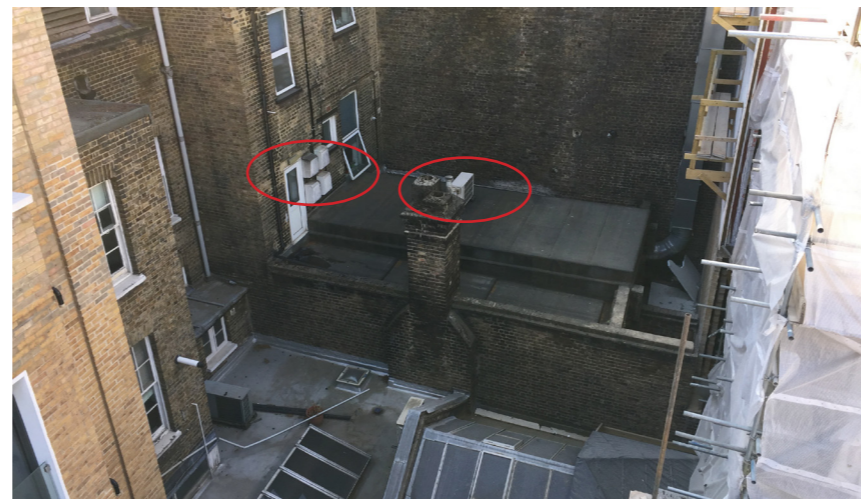
Fig 16. A/C plant for 37 Gray's Inn Road - without any acoustic enclosure - overlooked by all rear windows of adjacent properties
