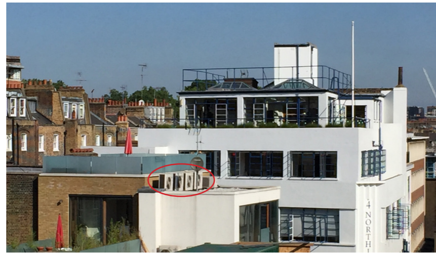
Fig 14. Rooftop A/C units at 12 King's Mews without an acoustic enclosure
