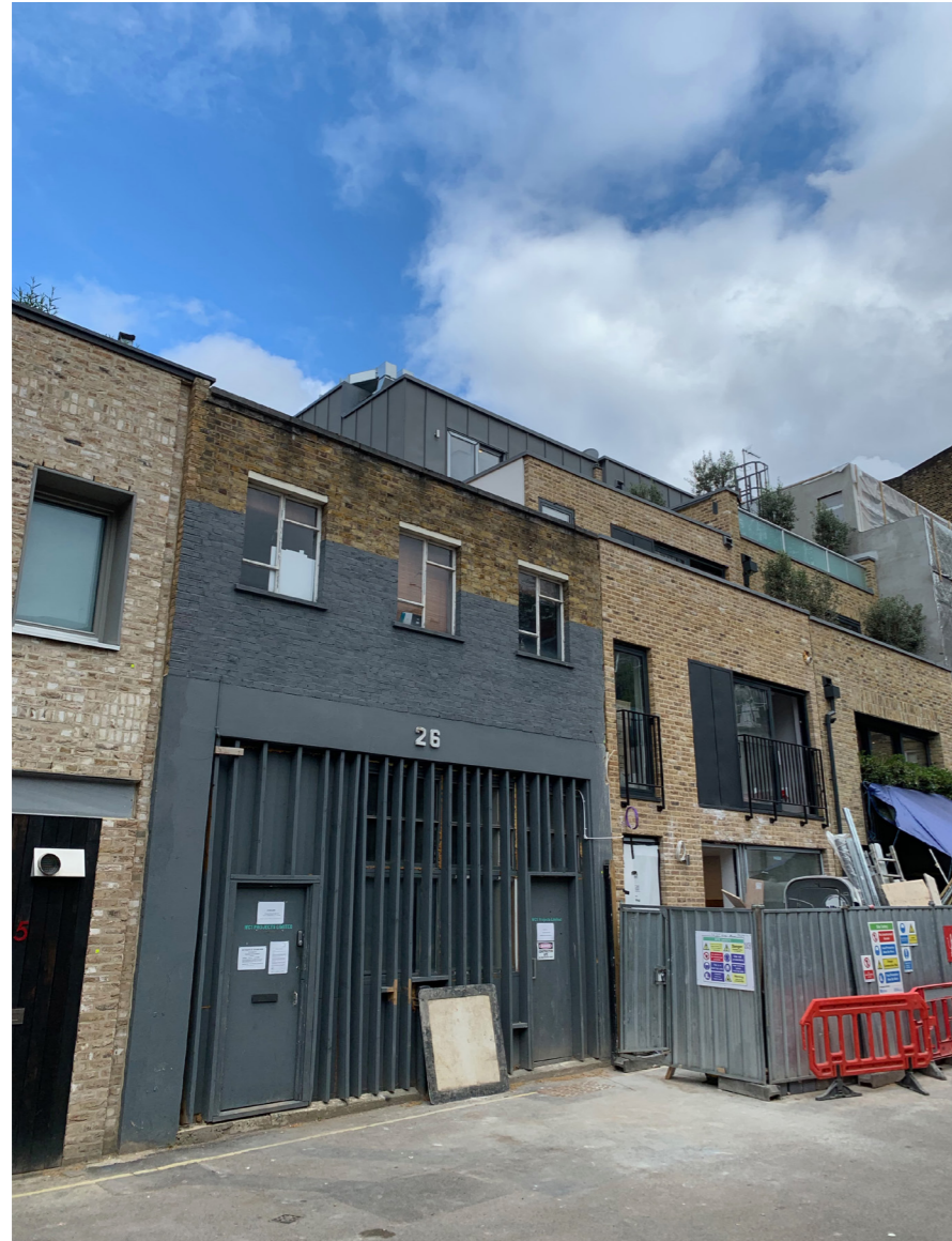
Fig 1. View of No. 27 King's Mews from the Mews. Works are currently in progress on no. 27 and adjacent buildings. From the Mews the only visible aspect of the additions that are applied for here is the corner of the air duct where it passes over the top of the lift shaft, currently seen as zinc but will be painted dark grey to match the roof finish.
