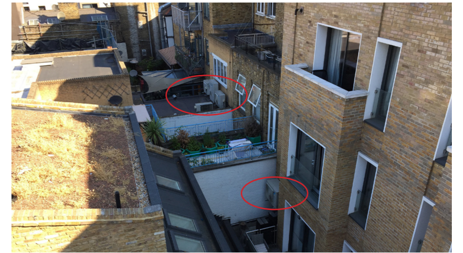
Fig 15. A/C plant for 34-49 and 47 Gray's Inn Road - without any acoustic enclosure - overlooked by all rear windows of adjacent properties
