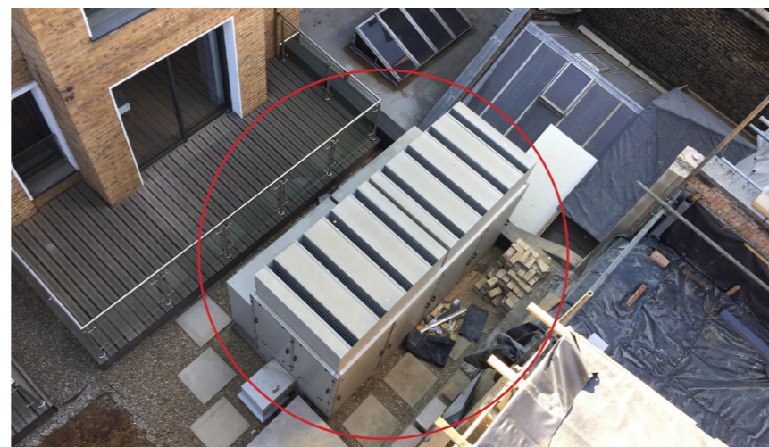
Fig 18. A/C plant for 34-49 Gray's Inn Road - overlooked by all rear windows of adjacent properties
