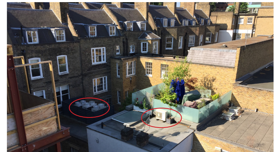
Fig 17. Rooftop A/C units at 1 King's Mews and 14 Theobald's Road without acoustic enclosures - overlooked by all rear windows of adjacent properties
