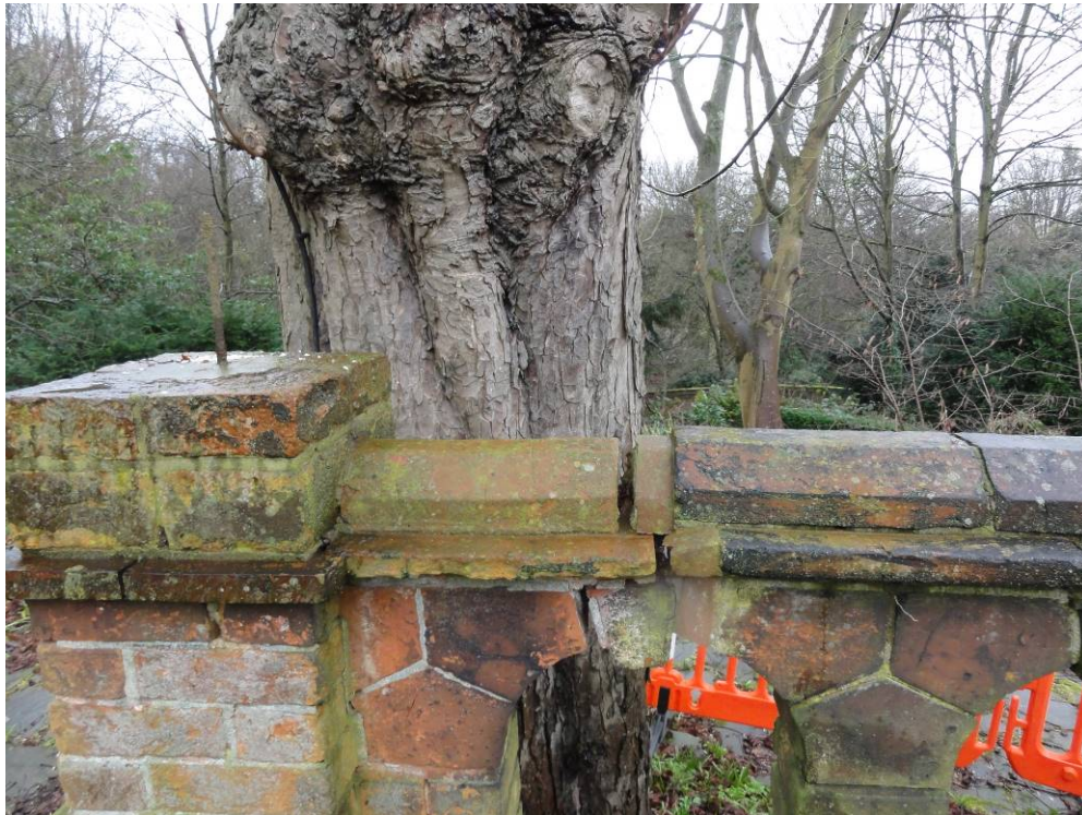
Photograph 11 – Damaged sections to top of balustrade.
