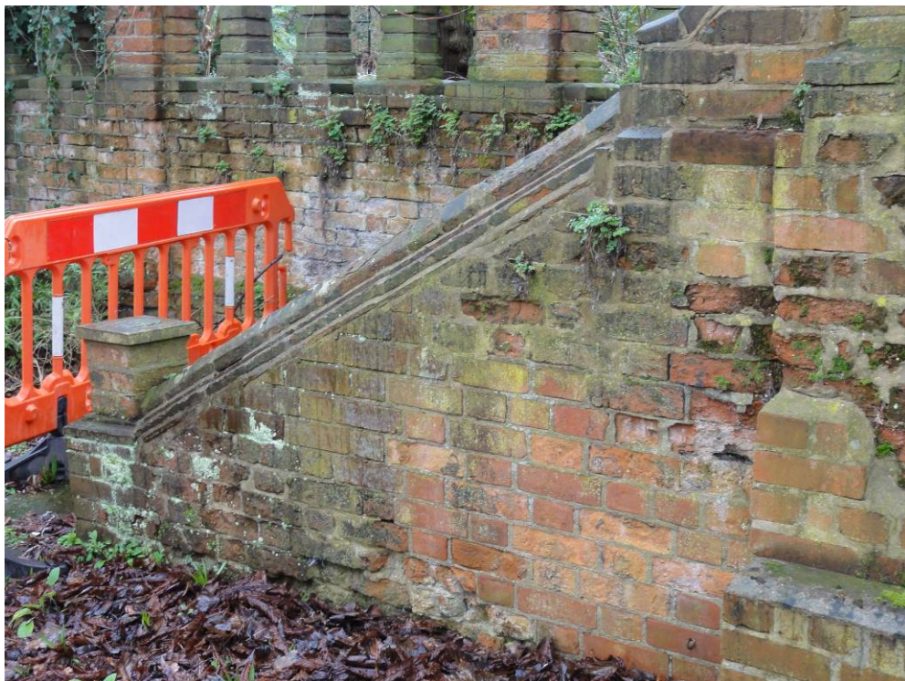
Photograph 6 – Spalled brickwork to stairs.
