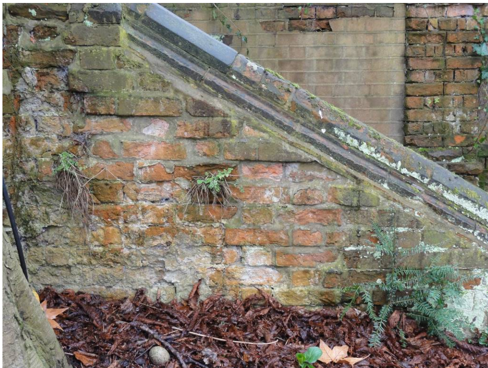
Photograph 4 – Vegetation to brickwork
