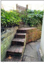
photo extract showing existing retaining garden wall and steps up to garden
