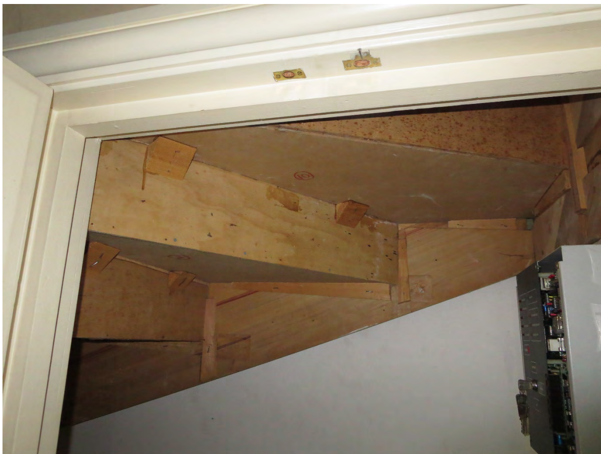
Image EDP 6: 2 Tower Court, representative view of the interior, showing the staircase has been replaced.
