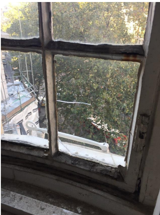
Plate 6: Windows in need of overhaul
