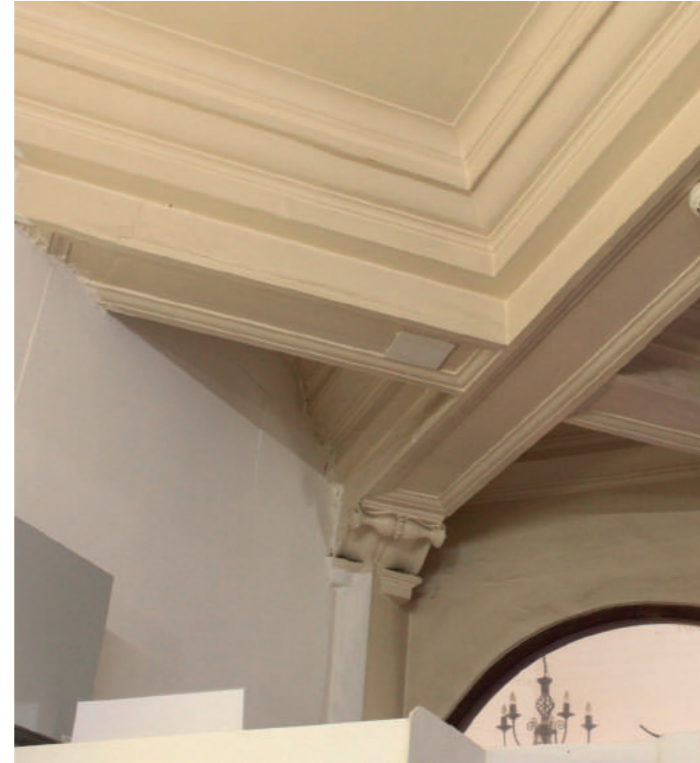
Non-original partition clashes with decorative ceiling
