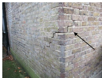
Cracking to rear right hand corner
