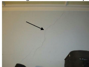
Cracking in flat 2 lounge to front of property
