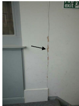
Cracking in communal hallway
