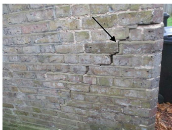
Cracking to rear right hand corner
