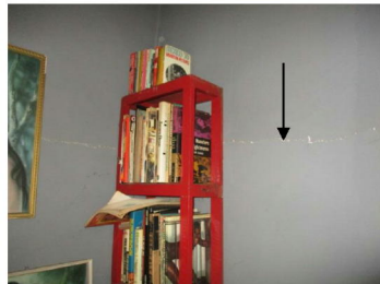
Cracking in flat 1 rear bedroom
