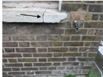
Cracking to rear
